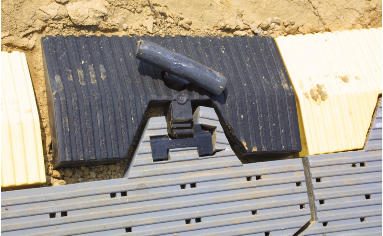
Photo 24. Isolated structural damage to SUPA-TRAC matting system at helipad edge
