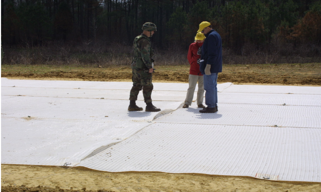
Photo 7. Completed Mobi-Mat helipad. (Note tops of pins used to hold it in place)
