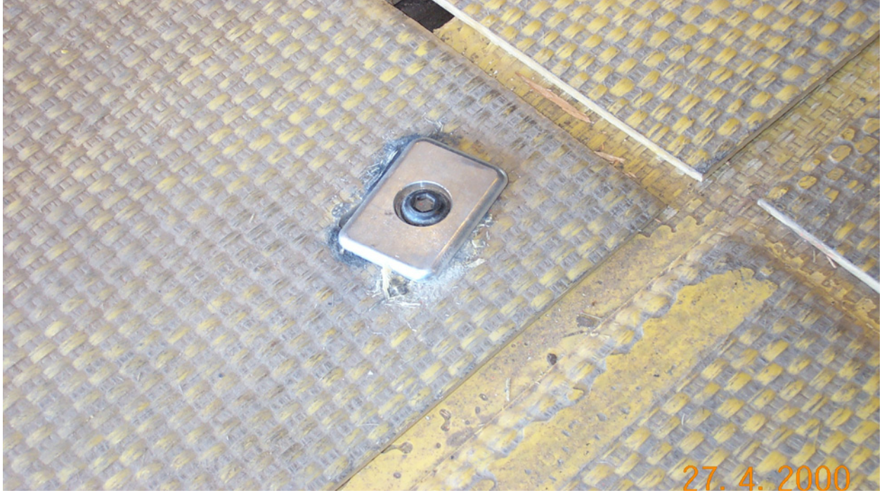
Photo 38. Movement of MP Mat pin within connection. Pin did not fail. (Low-strength soil, 3 to 5 CBR)
