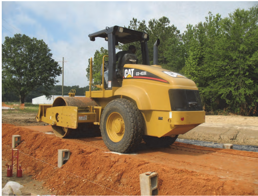
Figure 19. Caterpillar CS-443E vibratory roller used in soil compaction on SP-SM soil. Note string line and cinder blocks to provide thickness control.
