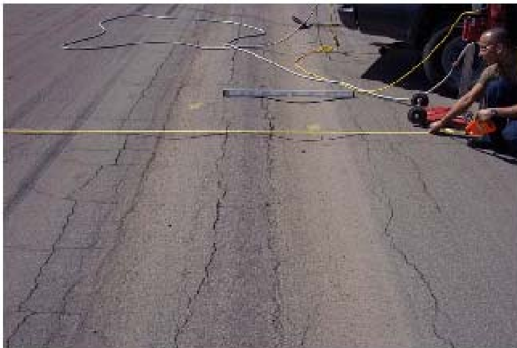
Figure A6. Runway asphalt distresses include cracking and rutting.
