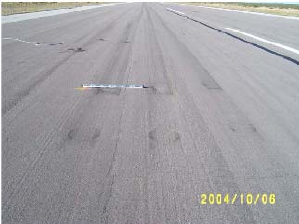
Figure A5. Rutting in asphalt with tire imprints – Runway 22 touchdown area.
