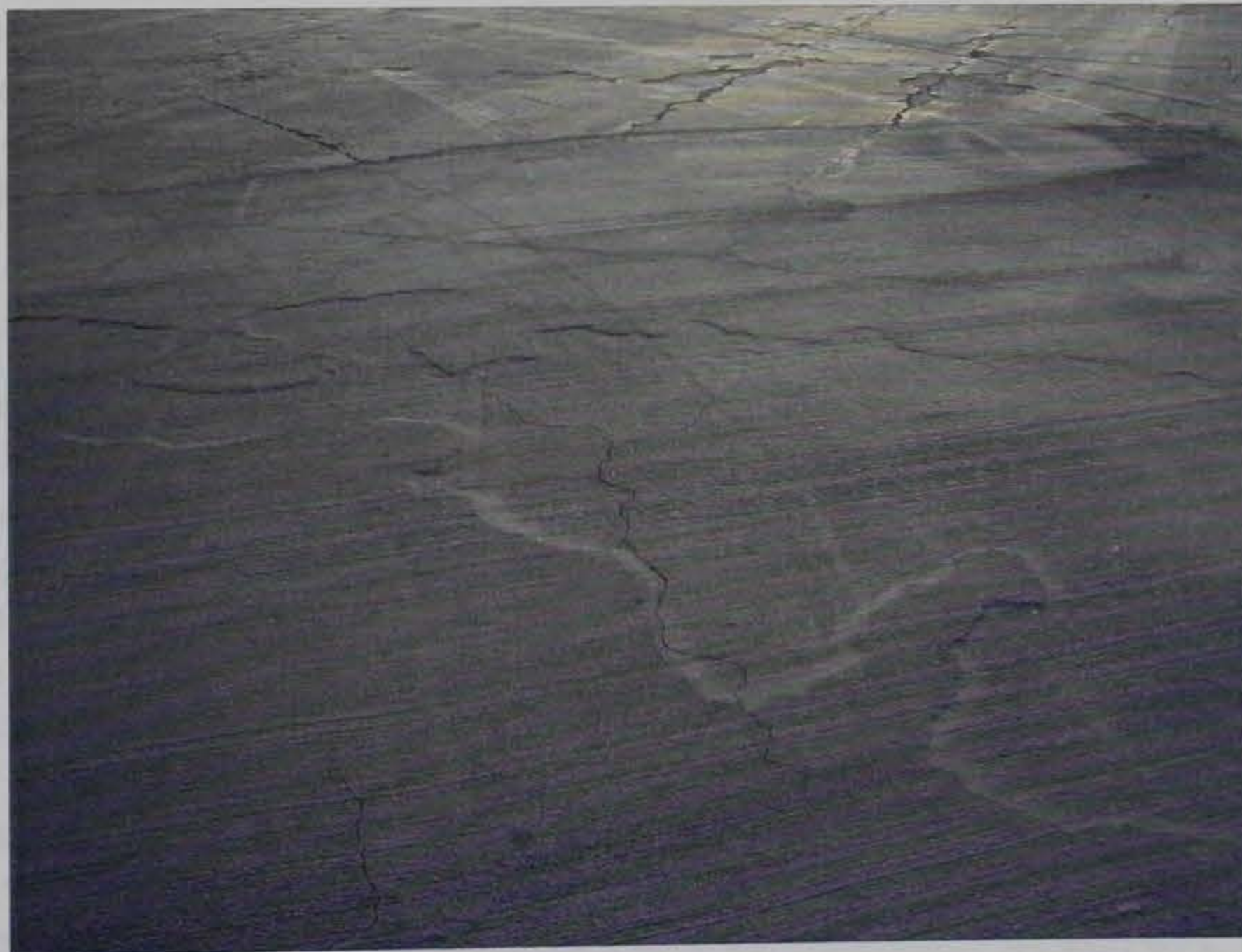
Figure 22. Area from Figure 20, about 2 years after E-Krete application. The large areas of missing coal tar have been completely encapsulated with no further delamination
