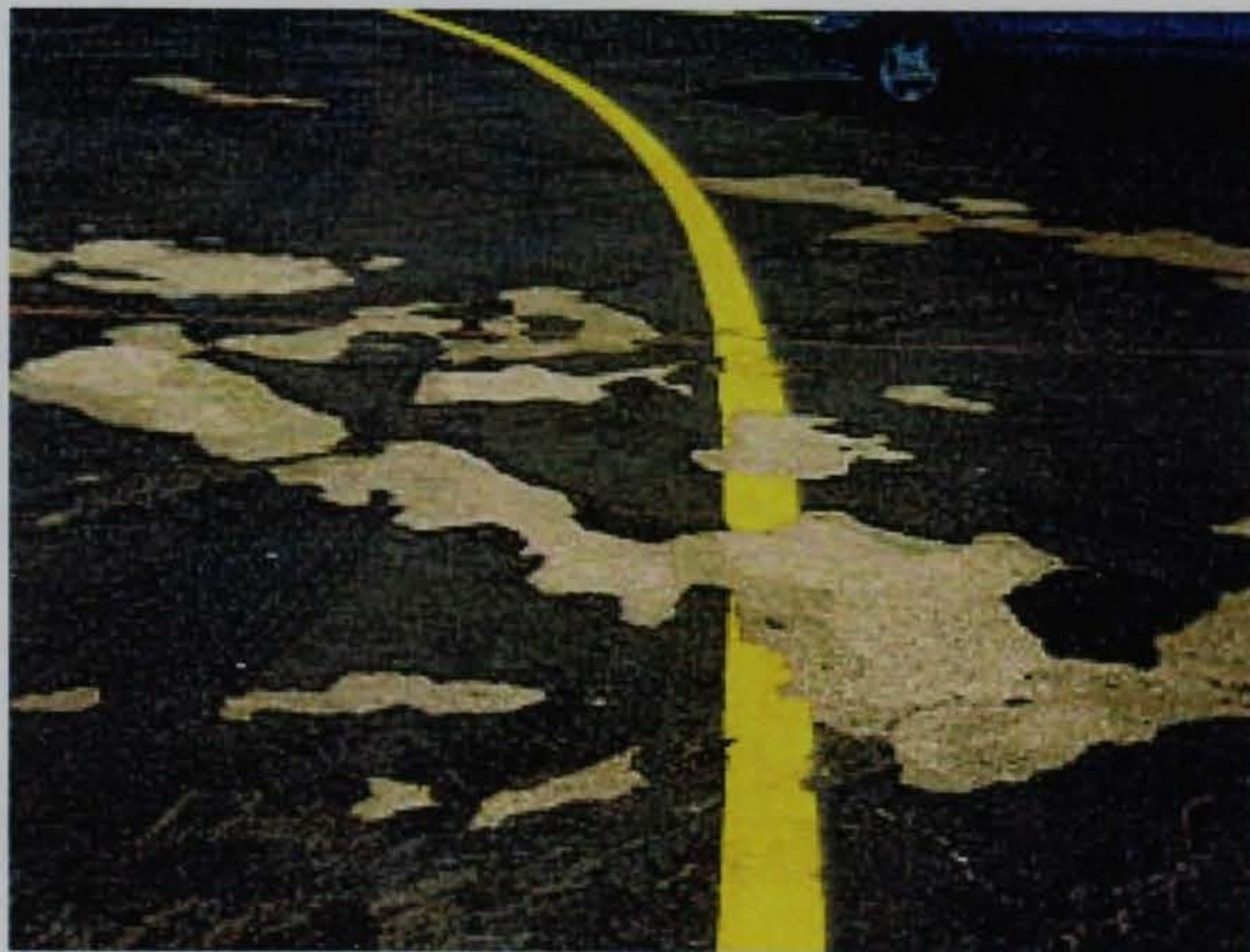
Figure 21. Severe delamination of existing coal tar surface (prior to E-Krete application)
