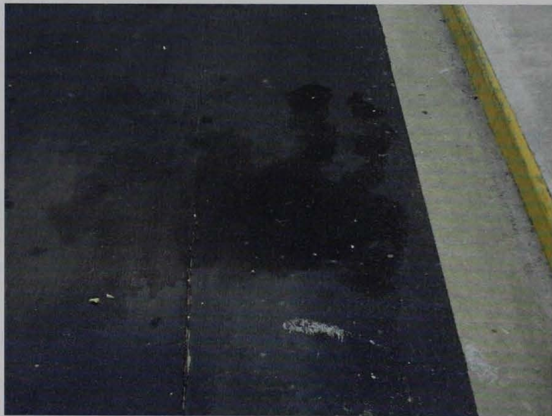
Figure 10. Oil staining of the E-Krete section at Tyndall AFB, October 2000
