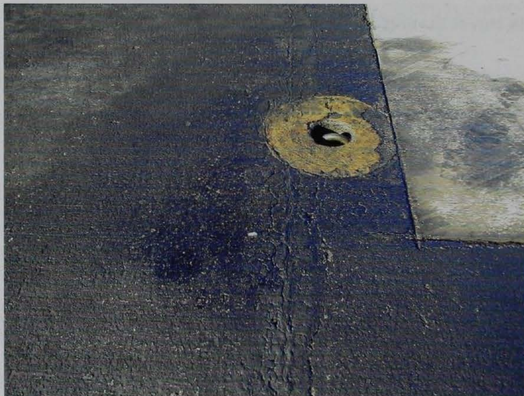
Figure 13. Closeup view of the E-Krete and PermaStripe at Norfolk Naval Station. The hydraulic fluid is literally pooled around the PermaStripe tie-down. Some delamination of the PermaStripe has occurred because of the ingress of hydraulic fluid under the surface of the PermaStripe where the asphalt and concrete meet
