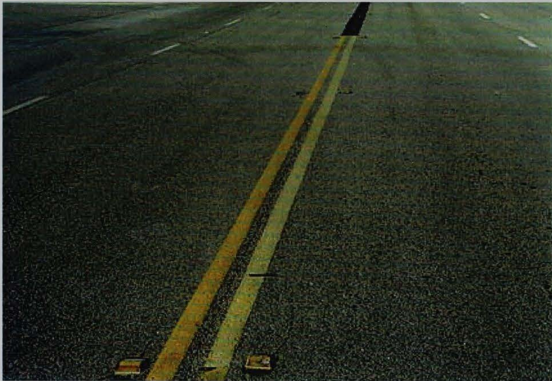
Figure 15. PermaStripe (on the left) roadway lines at Edwards AFB. The PermaStripe has not faded but is close to the original color as placed
