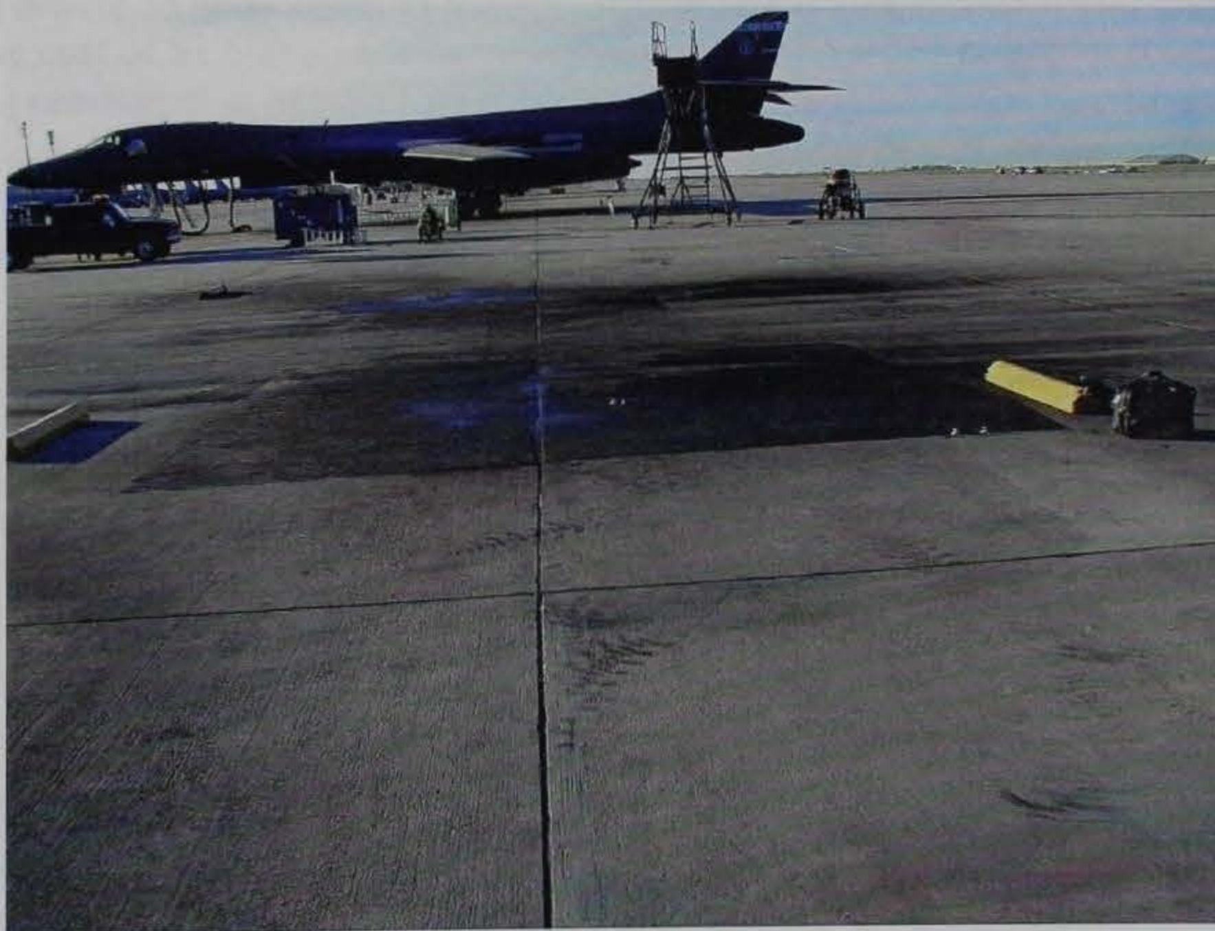
Figure 24. Overall view of B1B aircraft pad B10 in November 2000. As with B11, the E-Krete is completely soaked with aircraft hydraulic and turbine fluid and is in good condition.
