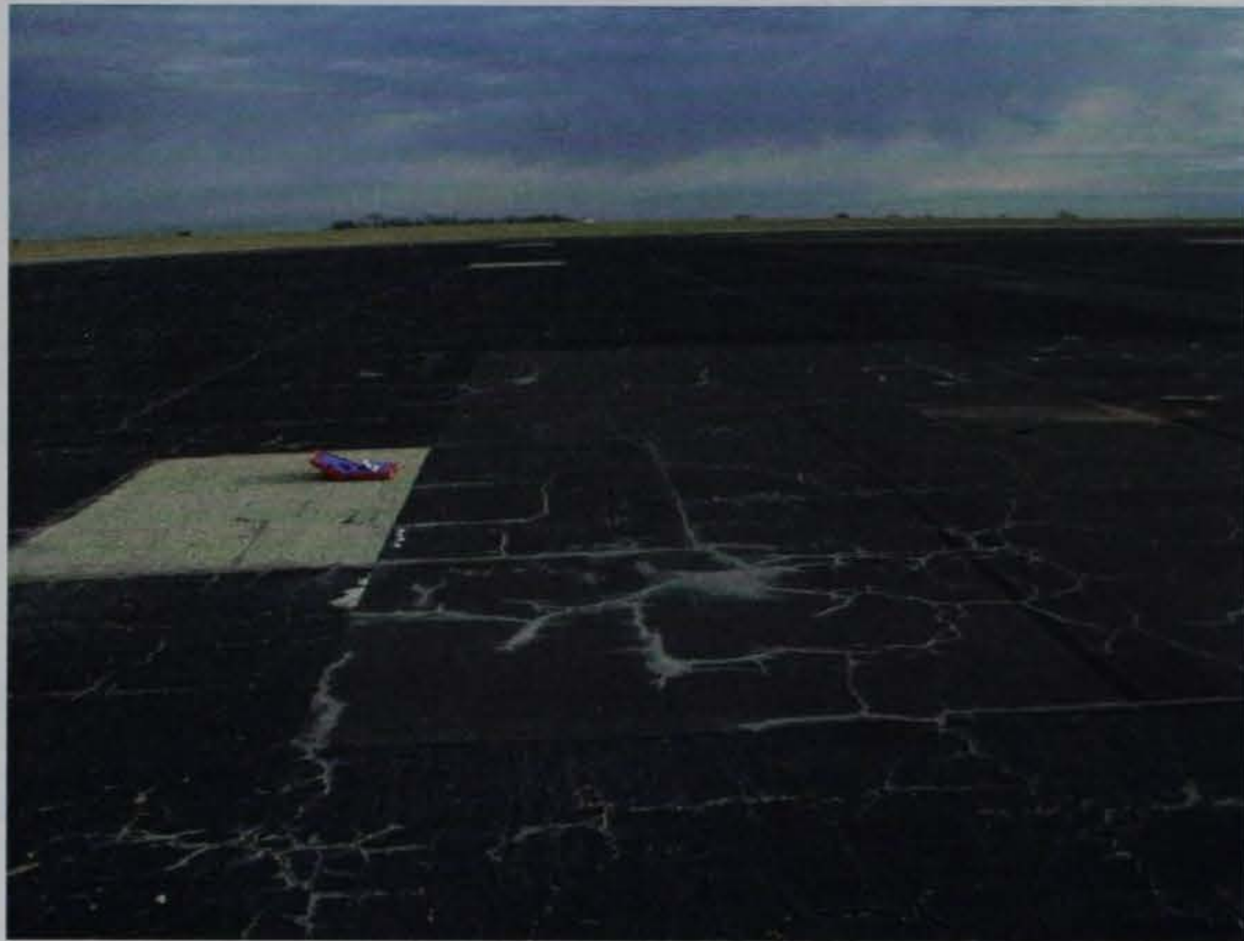
Figure 20. Large E-Krete section at Forbes Field. This section was placed on severely cracked coal tar and a portion of a small concrete island. The white staining about the reflective cracks is most likely effervescence from the cement powder within the E-Krete resulting from poor application conditions (see text for more detail).
