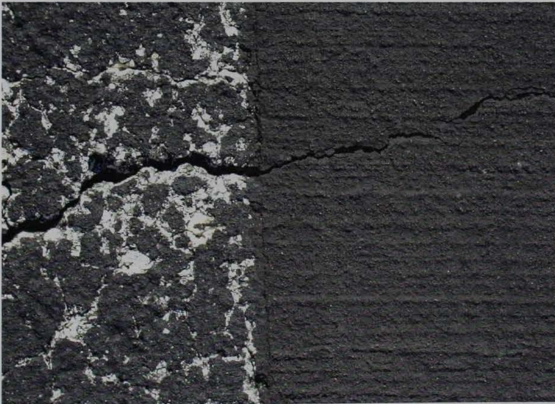
Figure 6. E-Krete section at MacDill AFB showing reflective cracking. Note that the crack has not widened or displayed any raveling from the crack face
