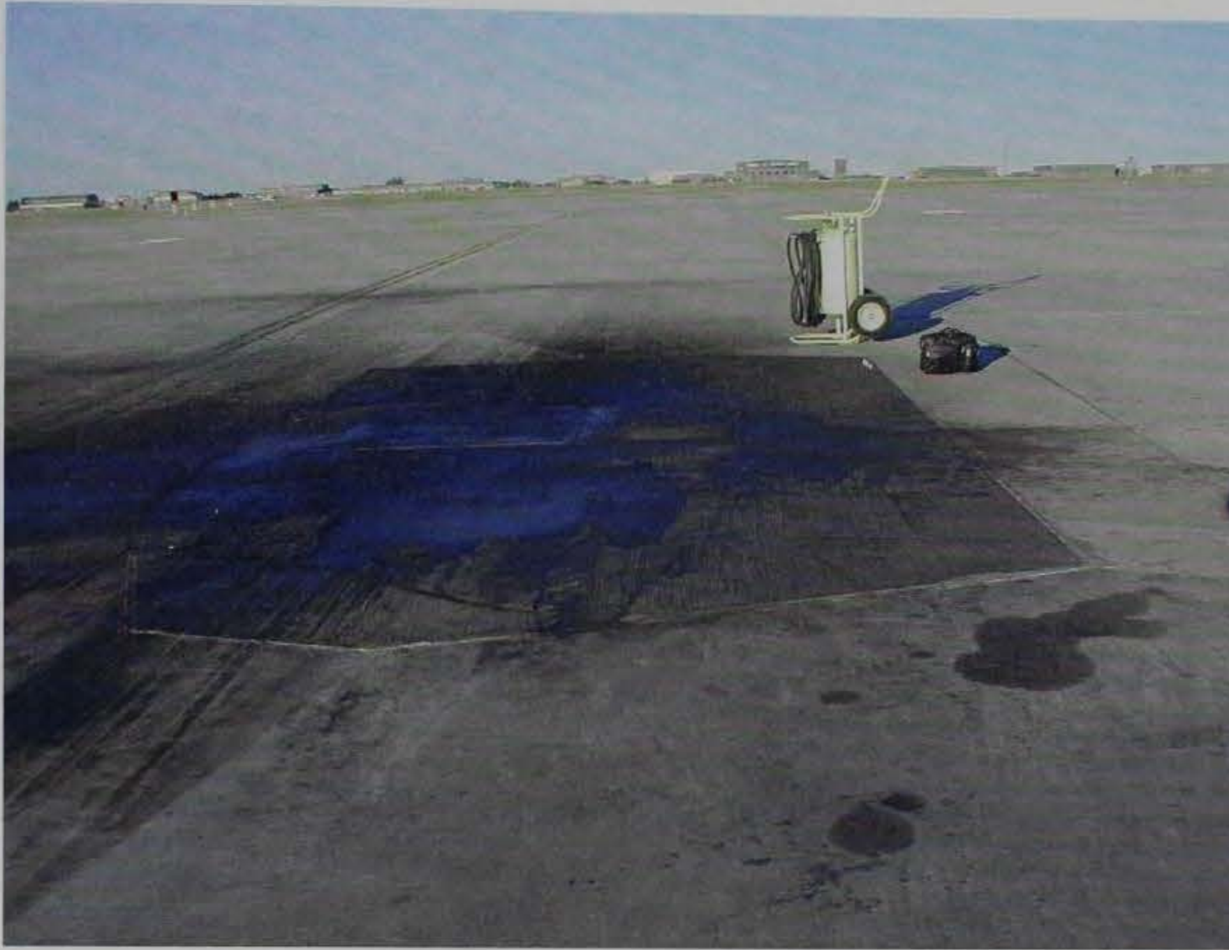
Figure 23. Overall view of B1B aircraft pad B11 in November 2000. The E-Krete is completely soaked with hydraulic and turbine fluid and is in good condition
