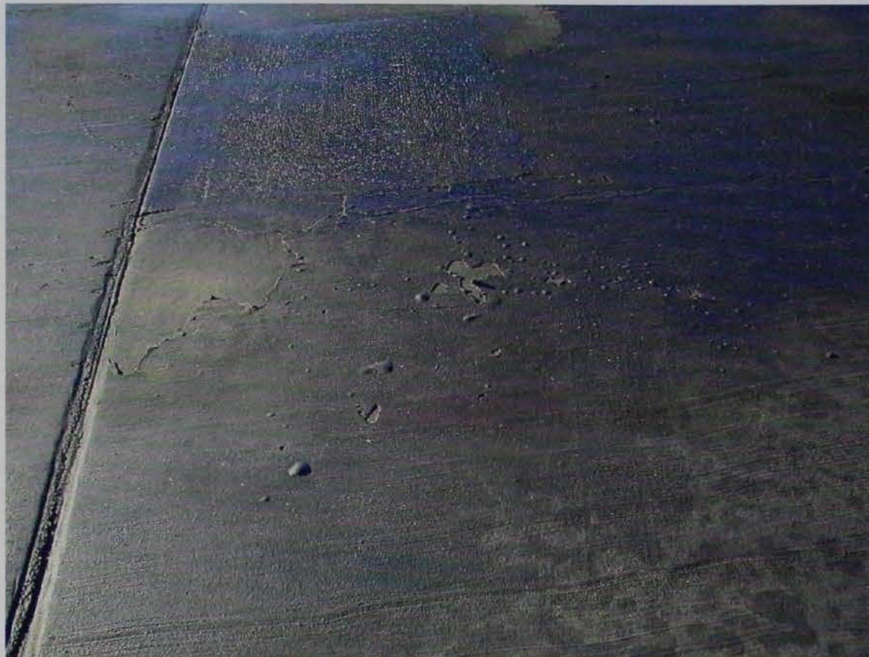
Figure 25. Closeup view of B-1B pad B11. On the left side of the joint, the E-Krete is intact but rubbery and has prevented ingress of aircraft fluid into the underlying concrete. On the right side of the joint, some delamination and blistering is evident. The delamination and blistering was likely the result of preexisting oil on the surface before application of the E-Krete
