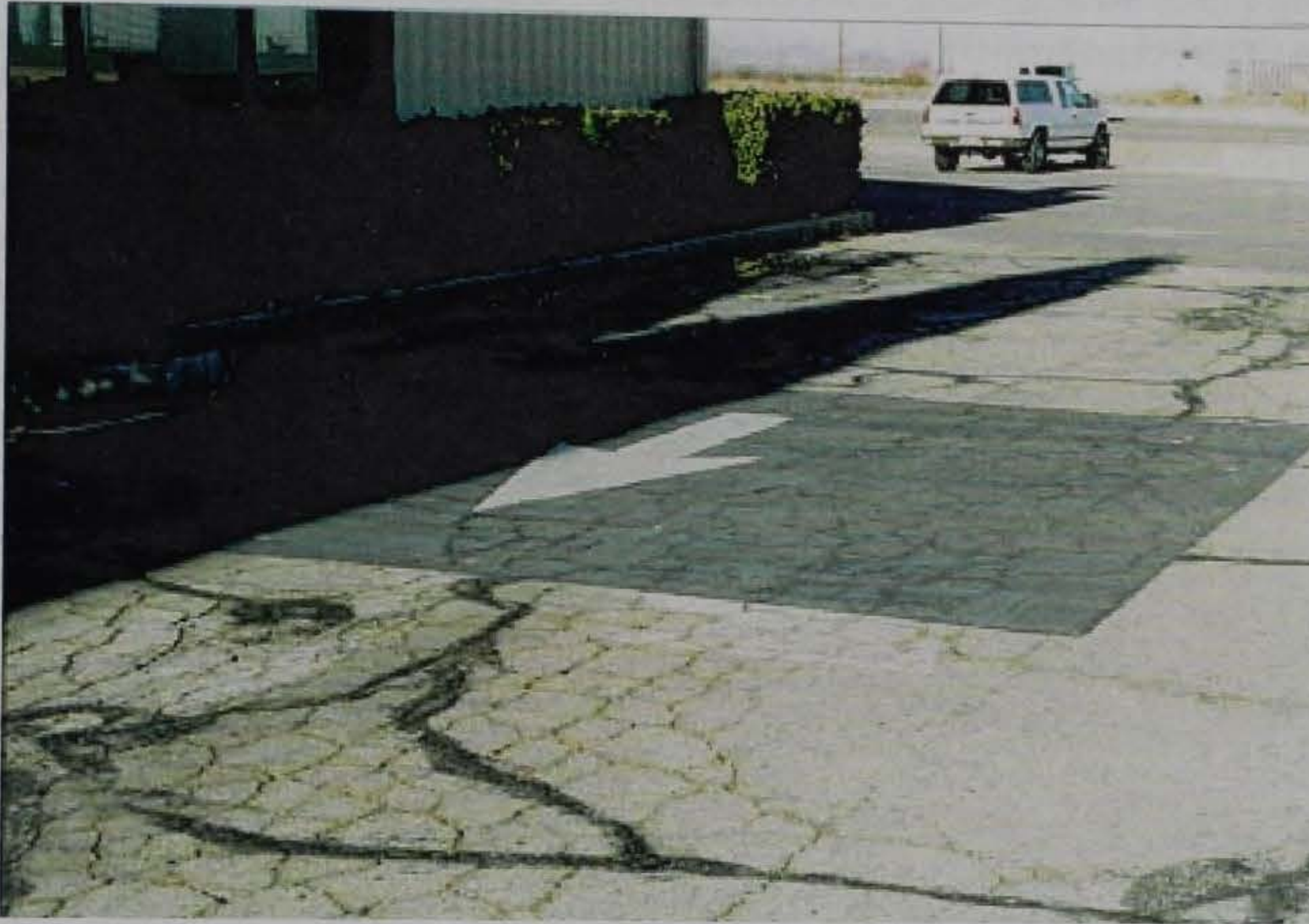
Figure 14. E-Krete and PermaStripe at Edwards AFB. Note the severely cracked asphalt surface upon which the E-Krete was placed. Although many of the cracks have reflected back up through the E-Krete, it is in much better condition than the asphalt with virtually no raveling, unlike the surrounding pavement
