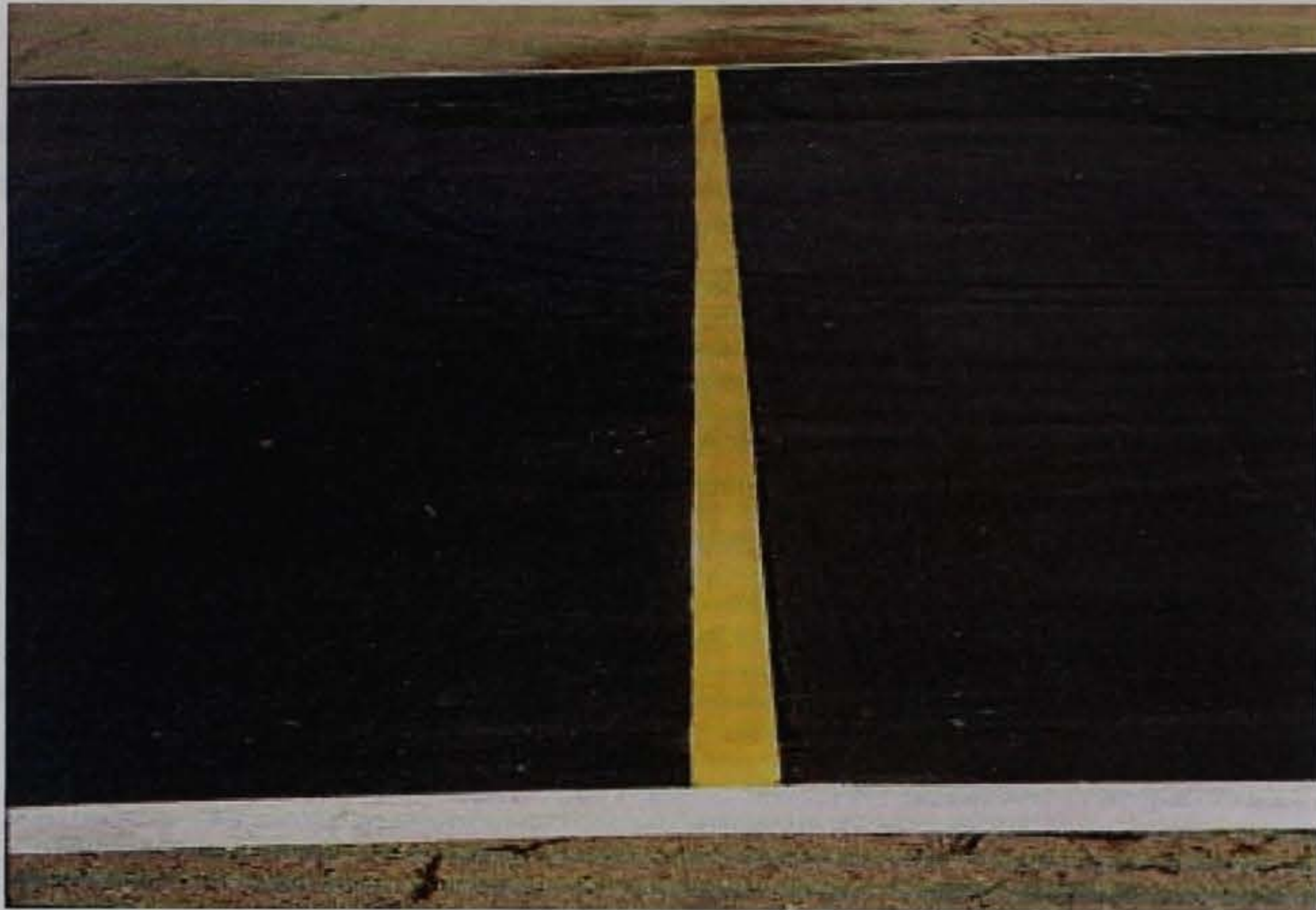
Figure 17. E-Krete and PermaStripe at North Island NAS. The PermaStripe has not faded and is holding its color well
