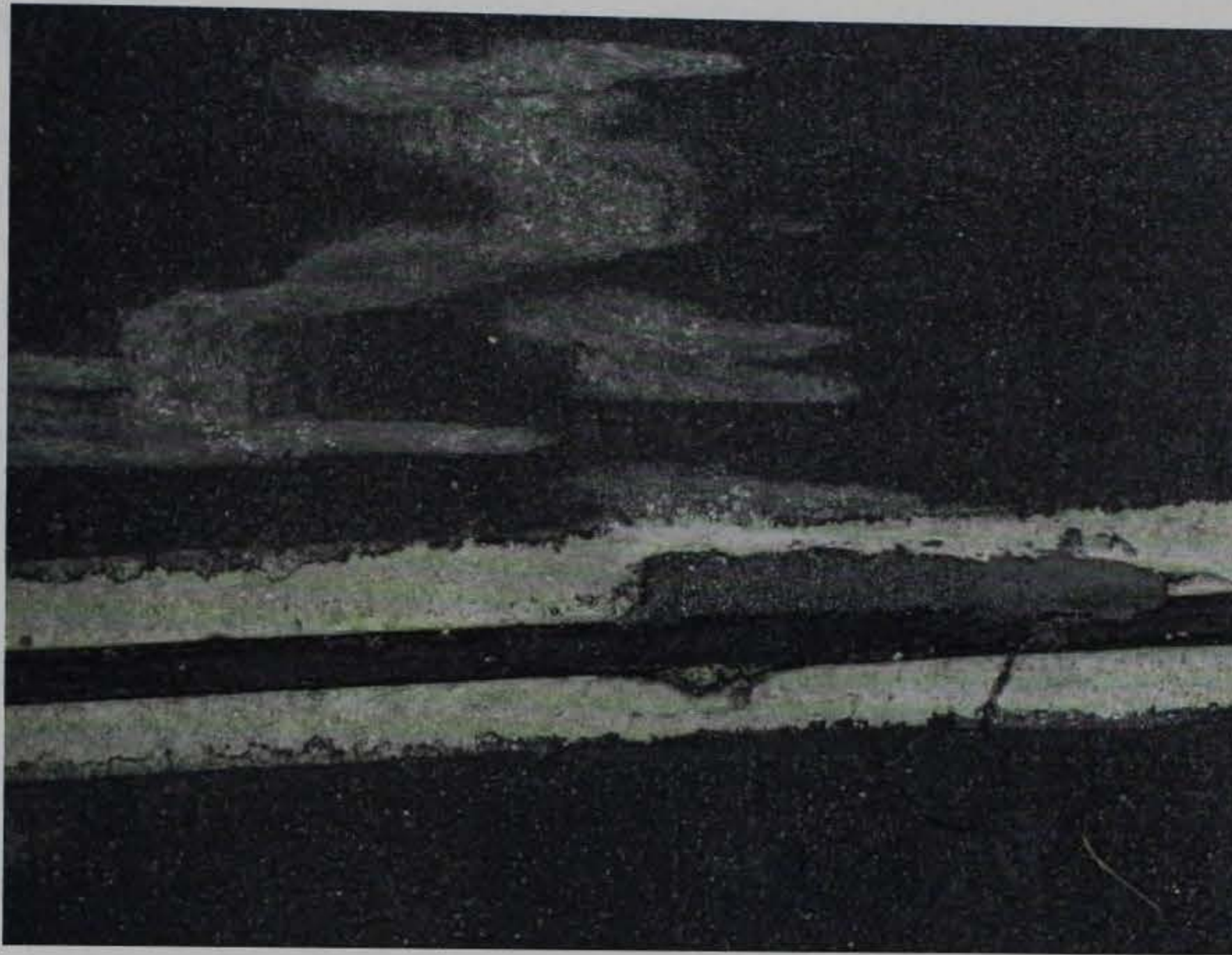
Figure 11. Scuff marks from backhoe stabilizers on the E-Krete section at Tyndall AFB, October 2000. The marks do not penetrate to the underlying cement
