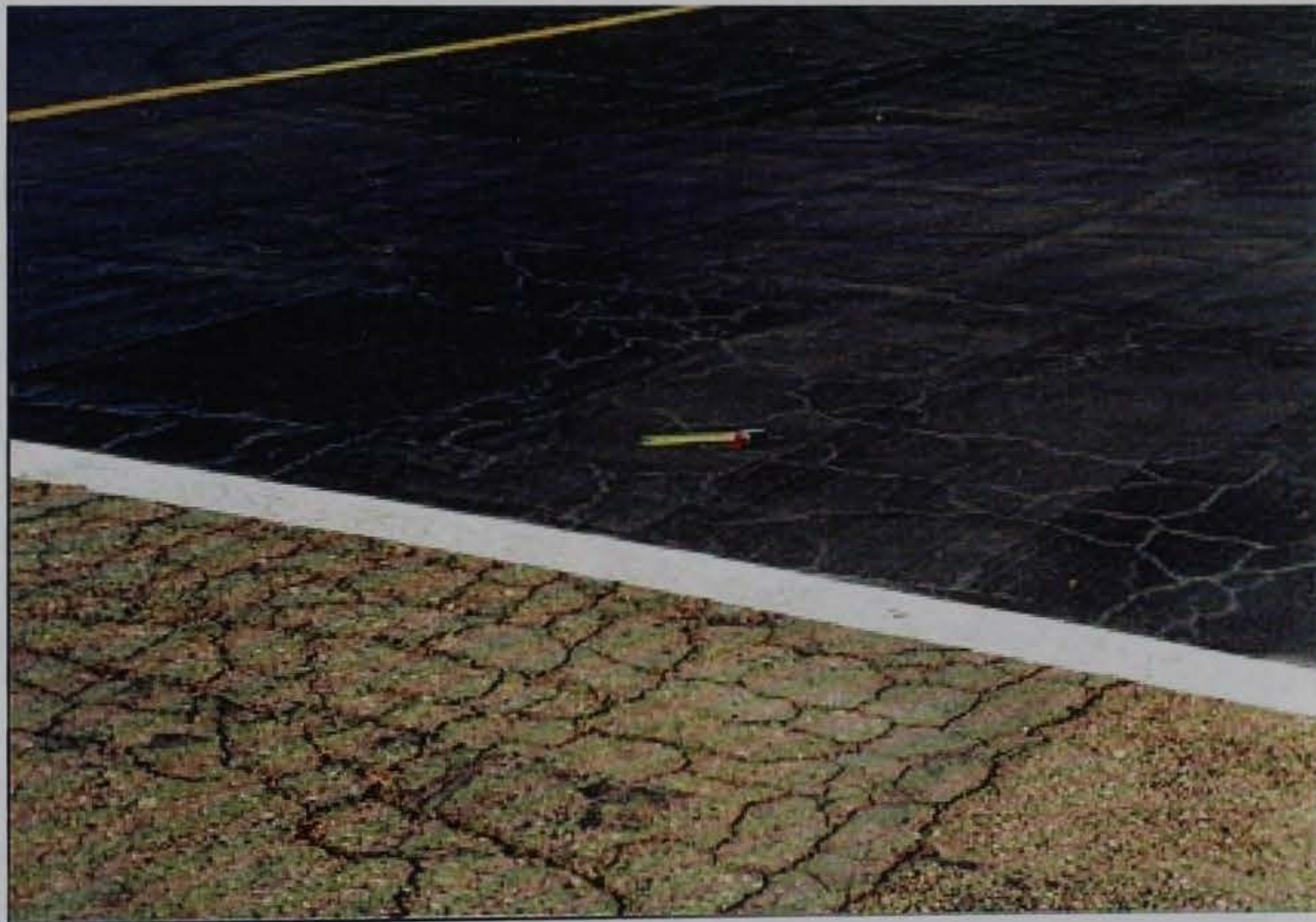
Figure 16. E-Krete and PermaStripe at North Island NAS. Note the severely cracked asphalt surface upon which the E-Krete was placed. Although many of the cracks have reflected back up through the E-Krete, it is in much better condition than the asphalt with virtually no raveling, unlike the surrounding pavement
