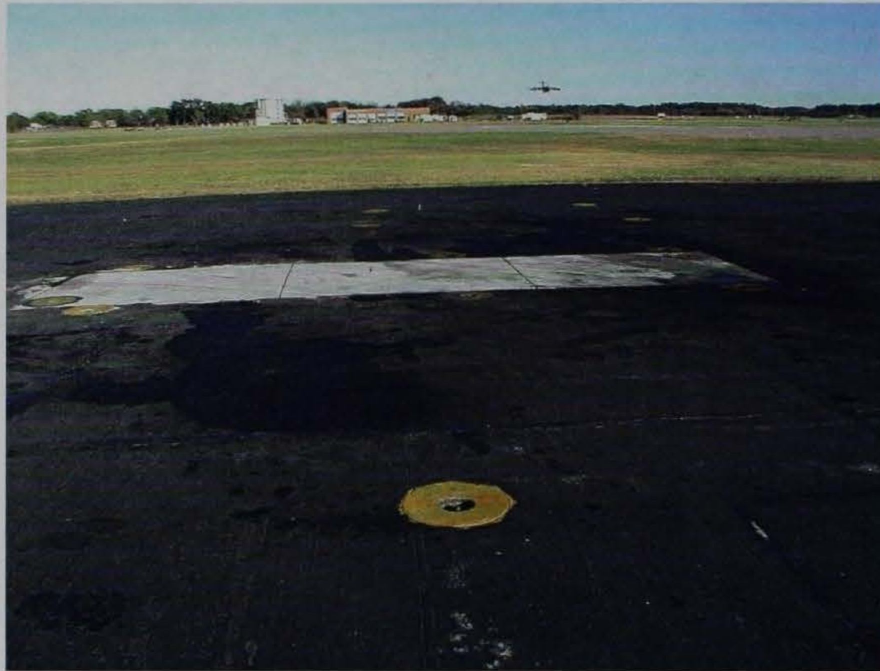
Figure 12. E-Krete and PermaStripe at Norfolk Naval Station. Note the severe hydraulic fluid staining around the concrete island. This area has been used repeatedly for servicing aircraft
