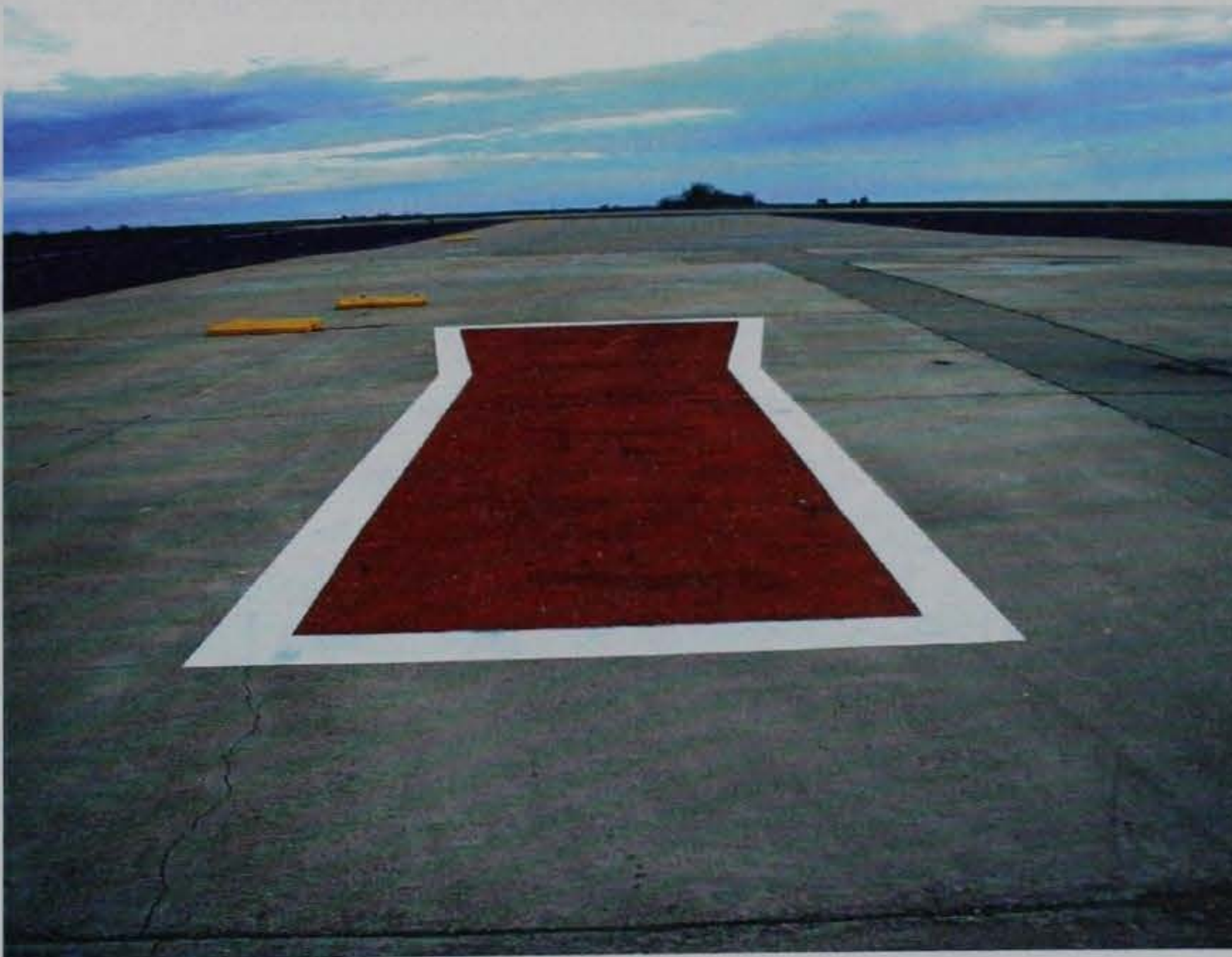
Figure 19. "Red Carpet" area in November 2000. Some fading of the red has occurred and reflective cracks are present, but overall, this section is in excellent condition
