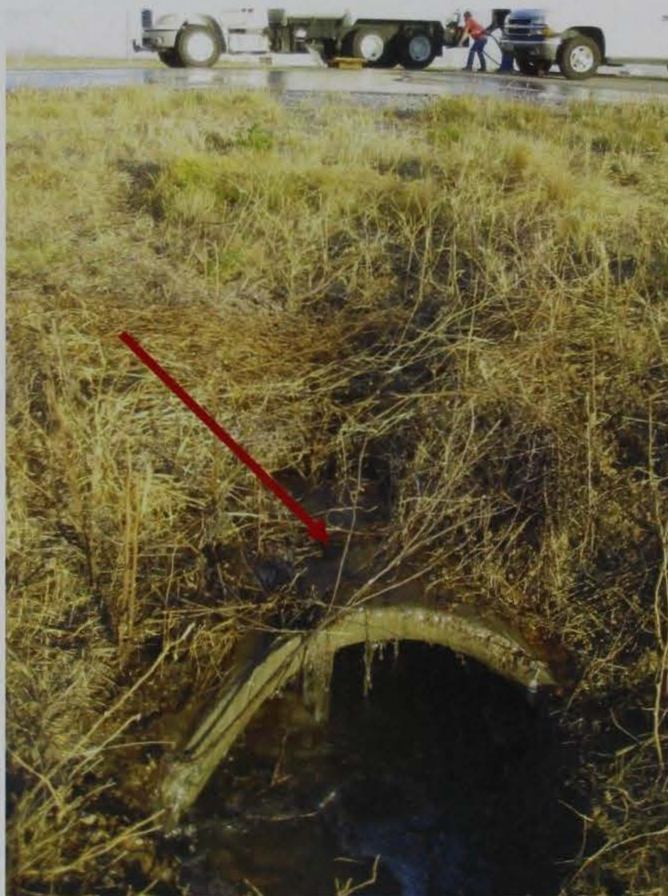
Figure 45. Surface drainage following path of drainage outlet pipe.
