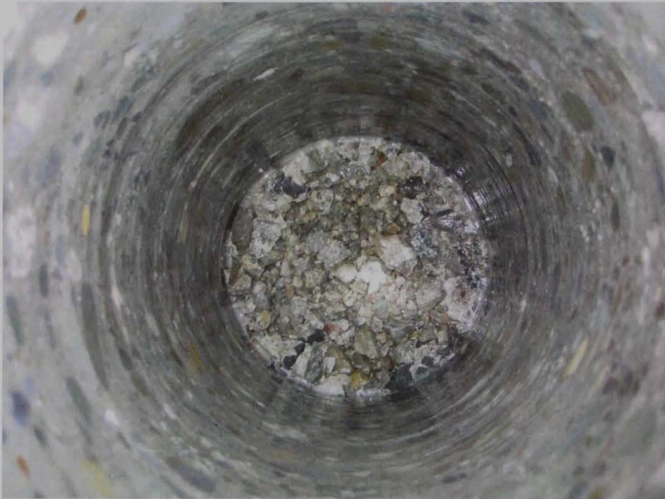
Figure 23. Rapid draining material beneath PCC at weather shelter apron.
