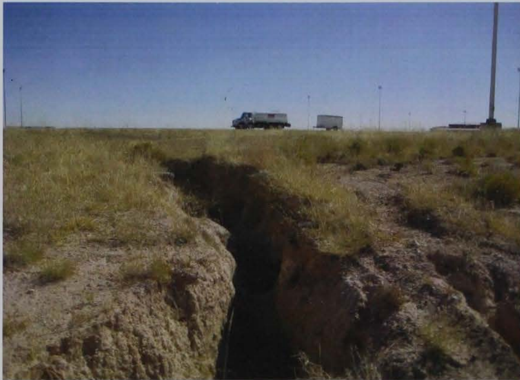
Figure 44. Soil erosion caused by surface water drainage.
