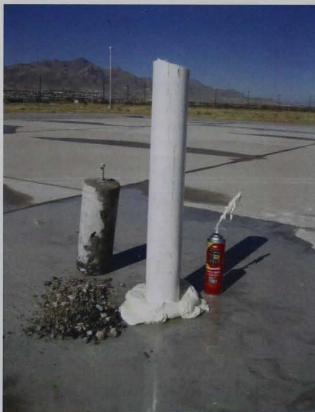
Figure 5. PVC pipe used to increase pressure head.
