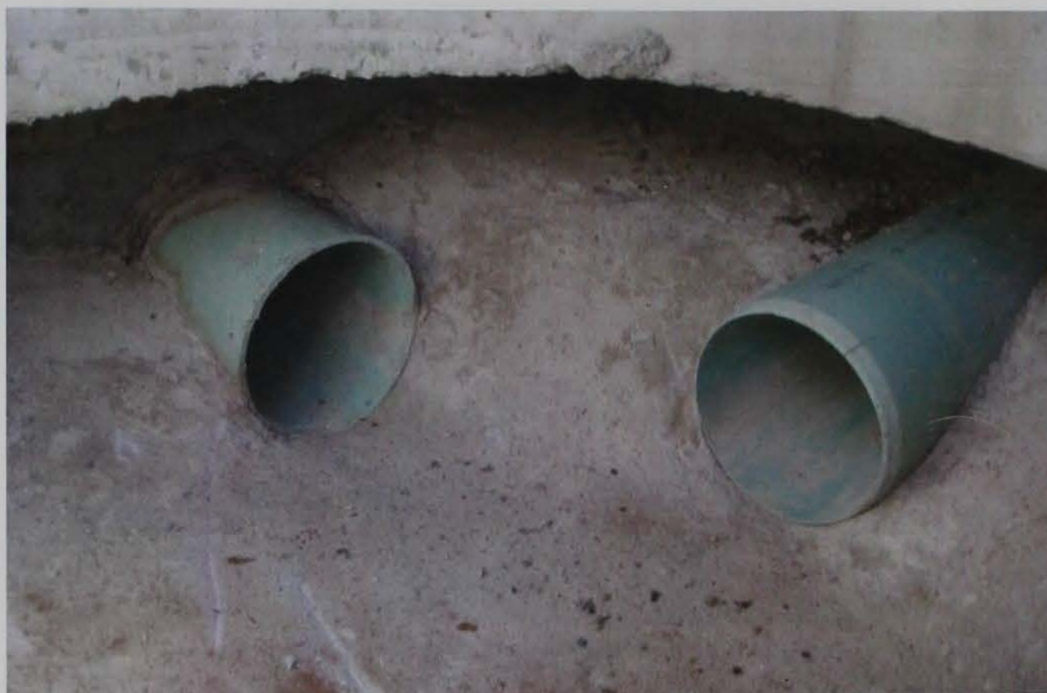
Figure 42. Drainage pipes converging at manhole on DAACG ramp.
