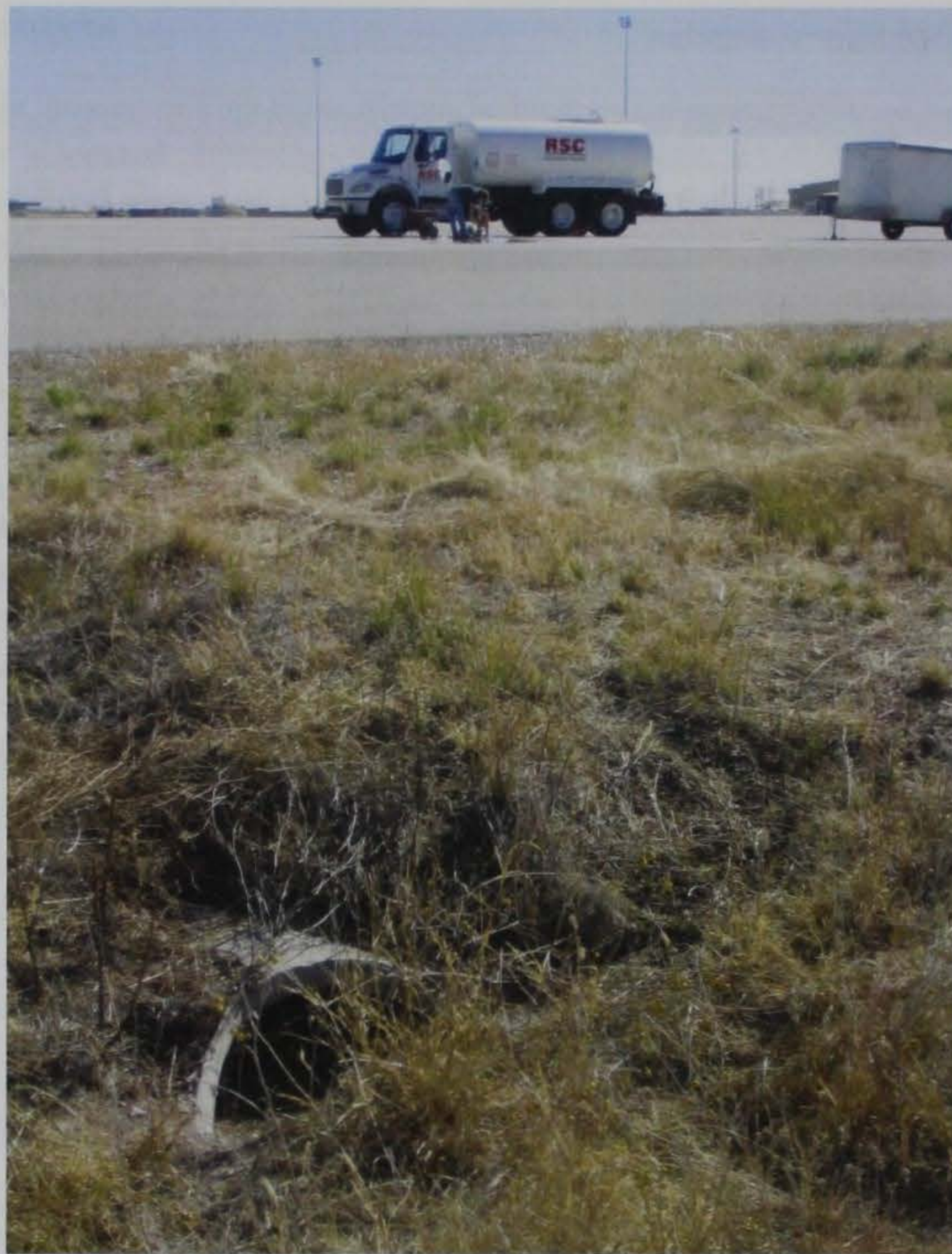
Figure 41. Poorly maintained outlet pipe leading from DAACG Ramp.
