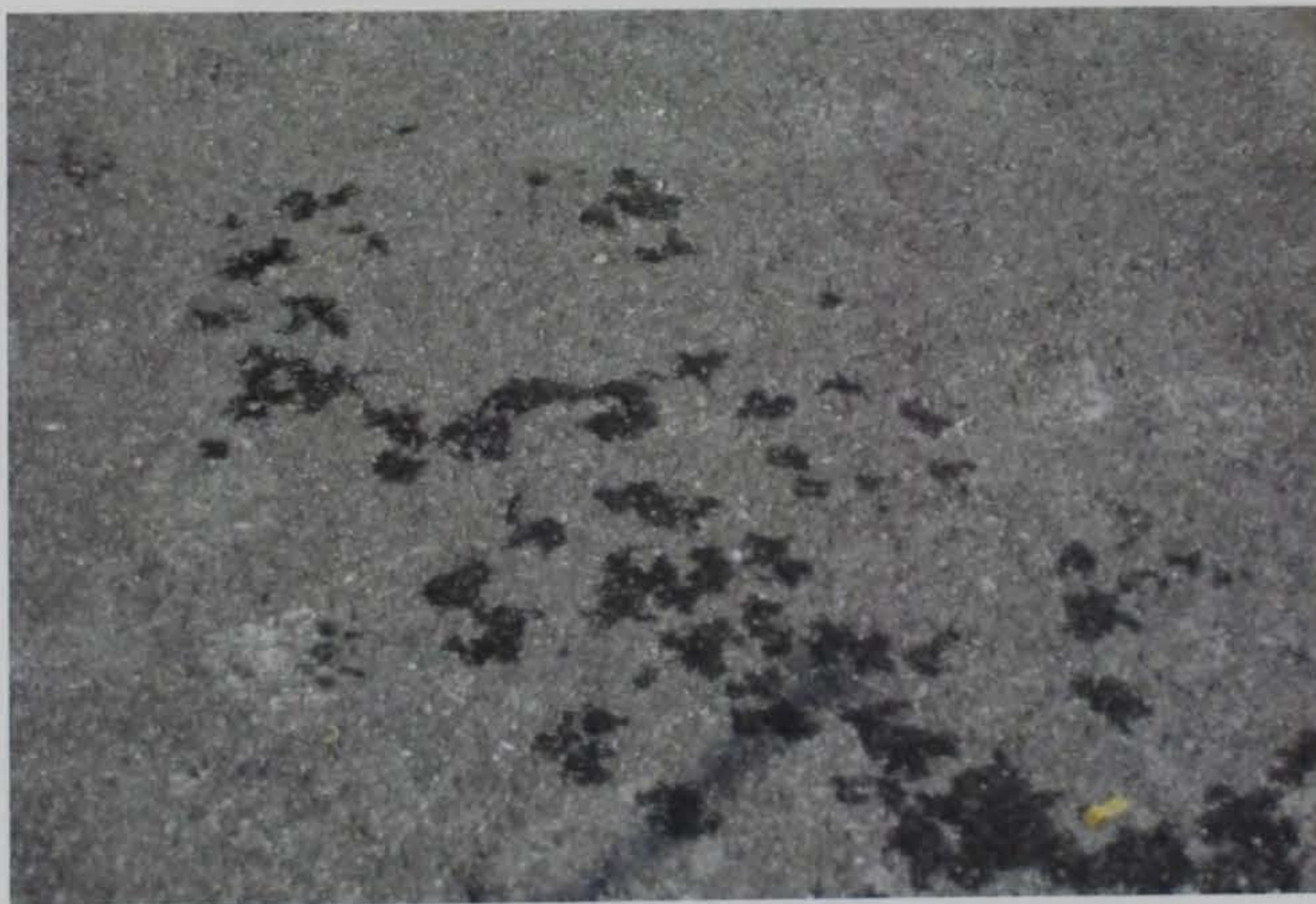
Figure 17. Water bleeding up through pavement on fuel cell taxiway.
