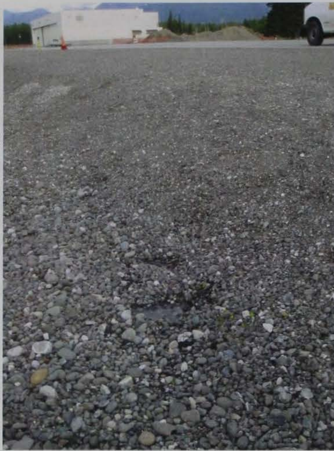
Figure 18. Water emerging from drainage layer on fuel cell taxiway.
