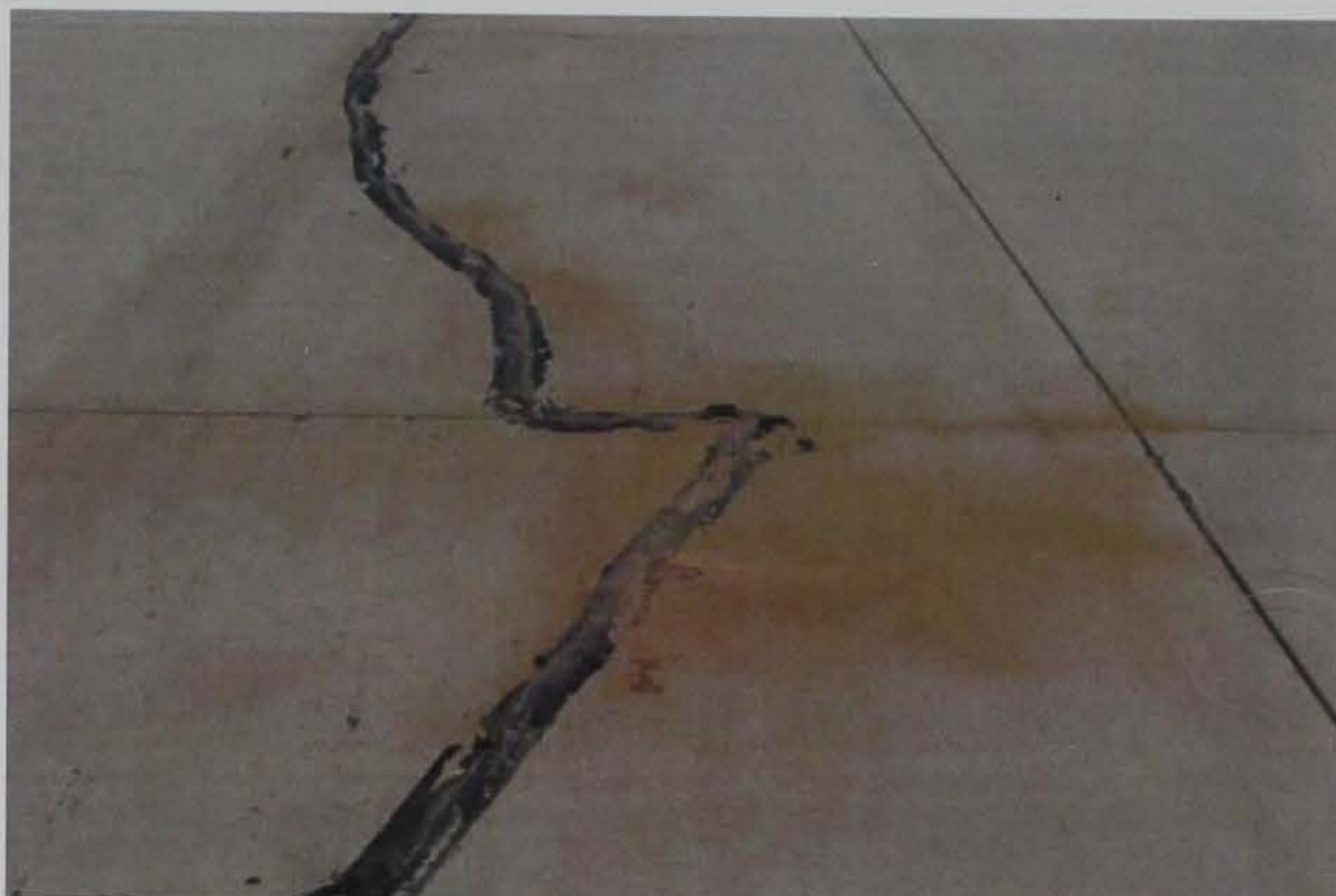
Figure 27. Staining from pumping due to inadequate base course material.
