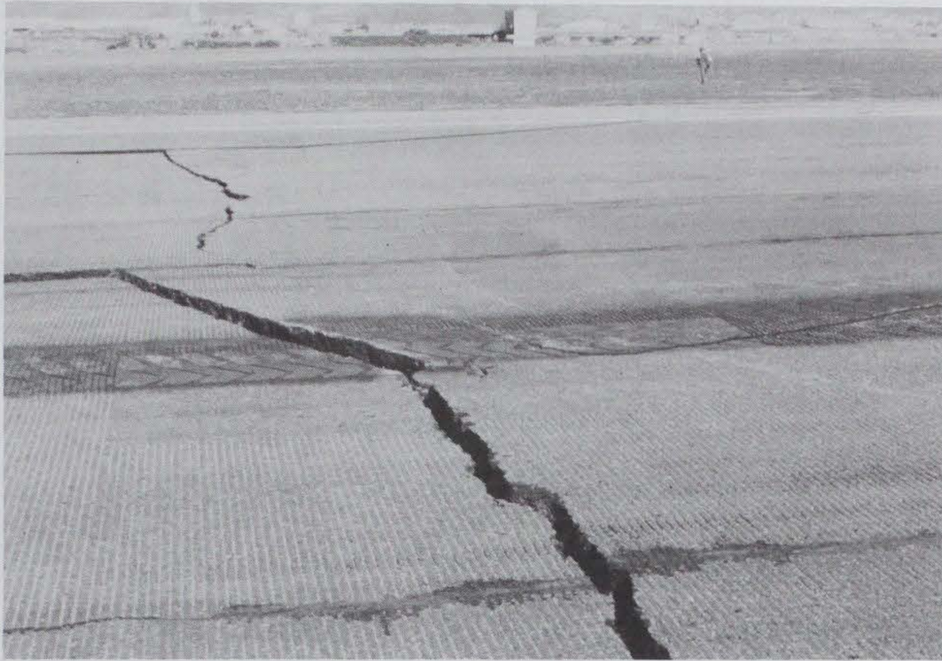
Figure 10. Transverse crack not following construction joint
