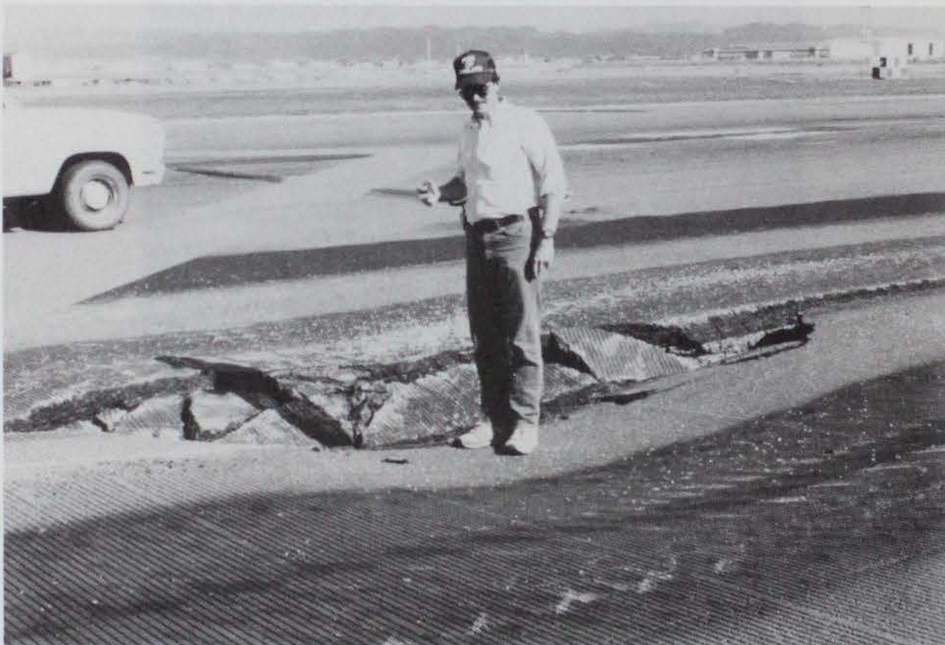
Figure 21. Pavement broken by proof roller adjacent to crack
