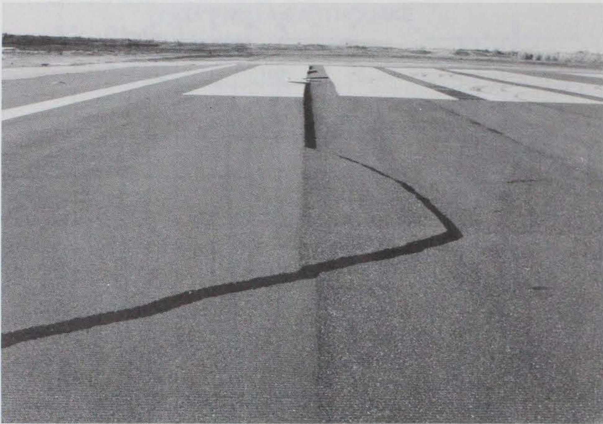
Figure 8. A view of crack following construction joint
