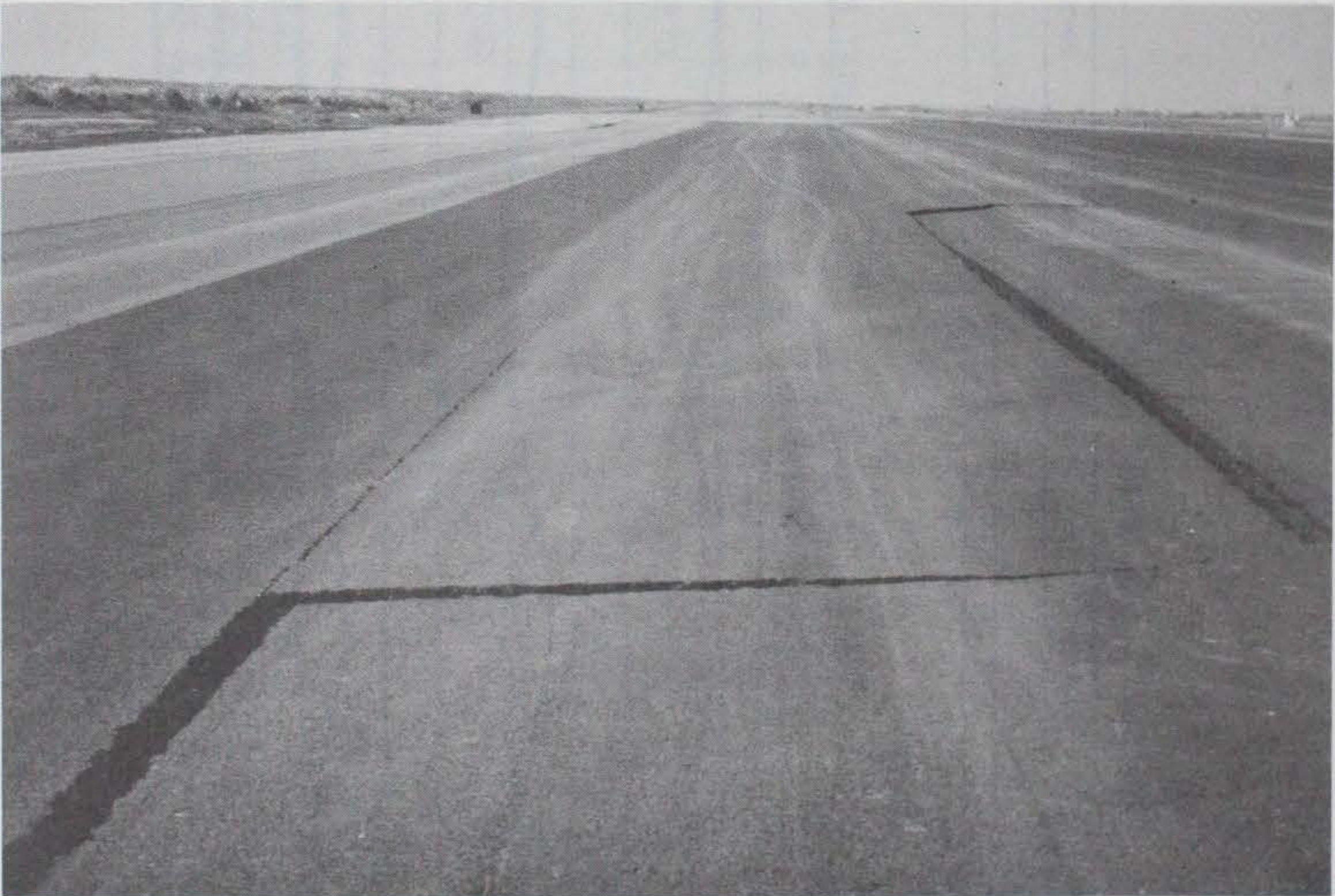
Figure 9. Close-up of crack following construction joint
