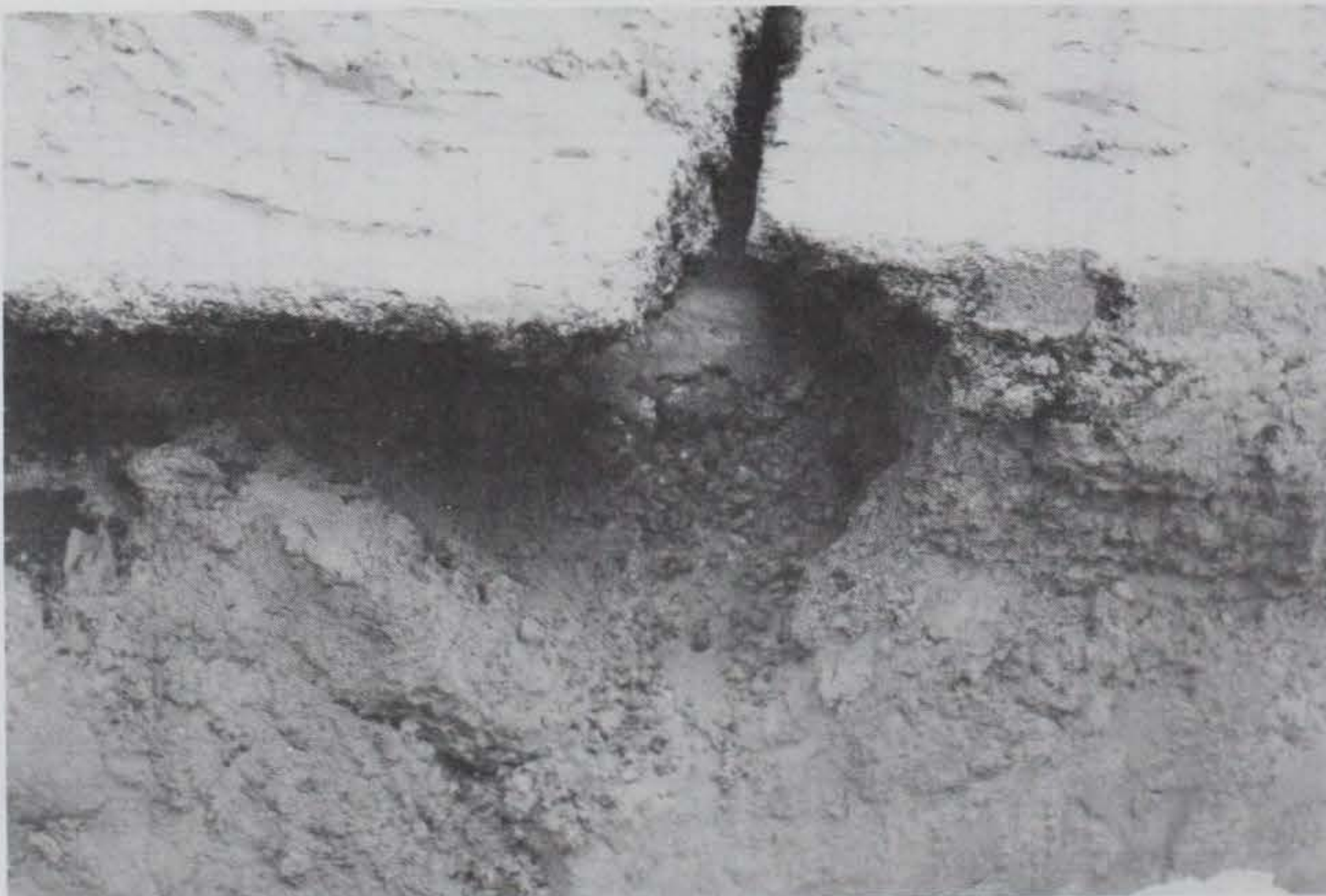
Figure 18. Void under AC pavement next to crack
