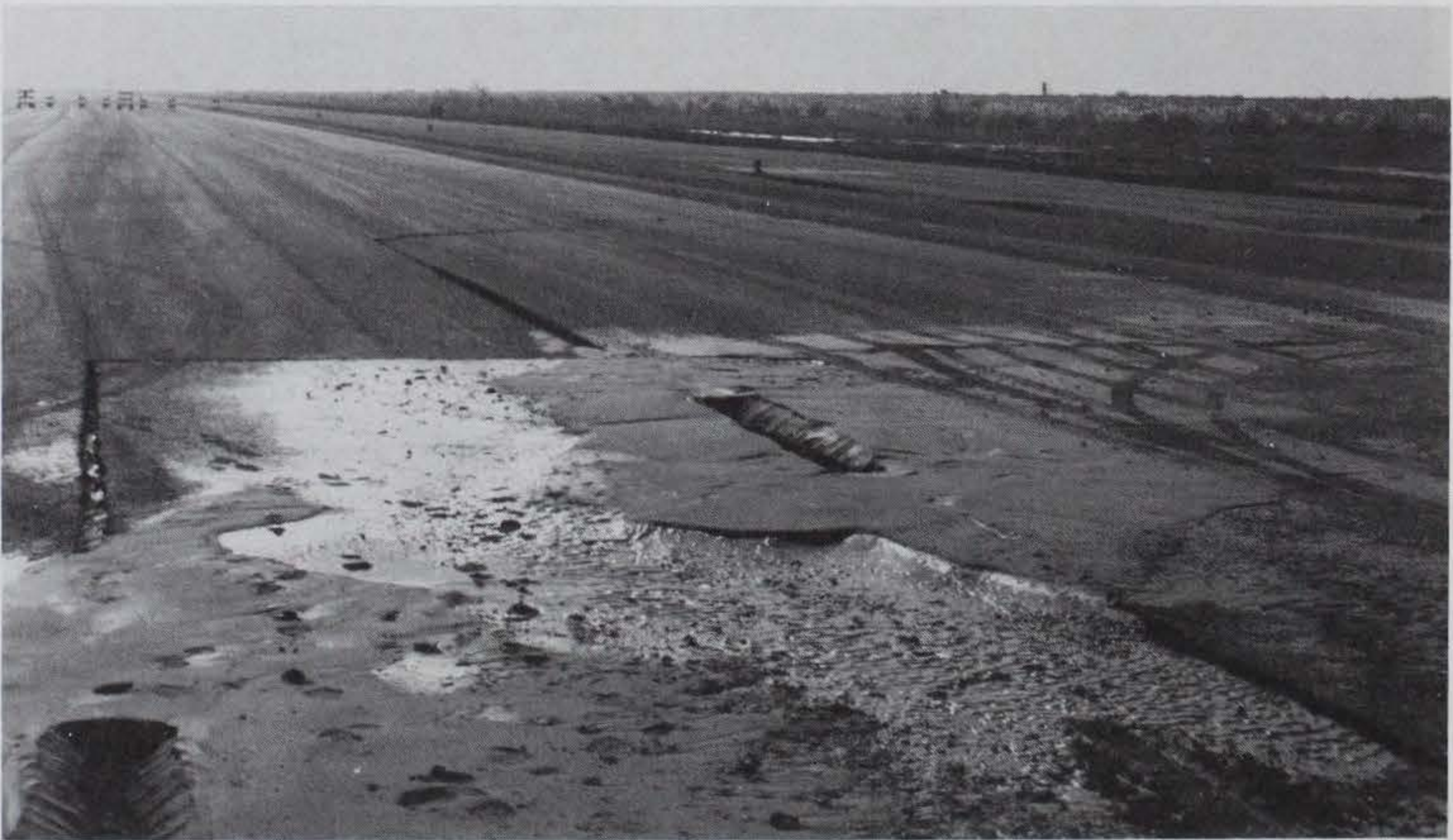
Figure 13. Overall view of sand boil on Runway 11-29
