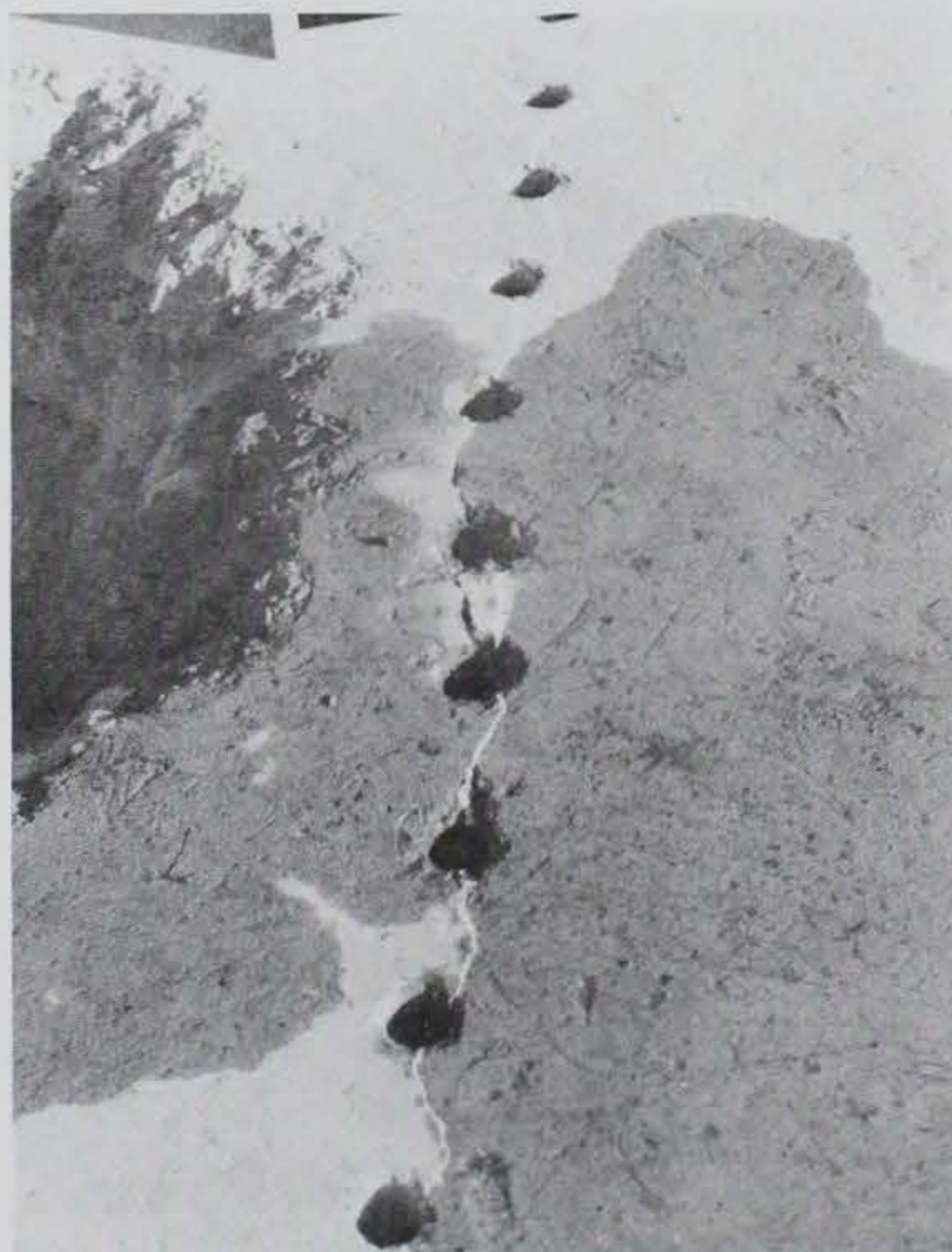
Photo 17. Extent of cracking and spalling existing after test 1, shot 6
