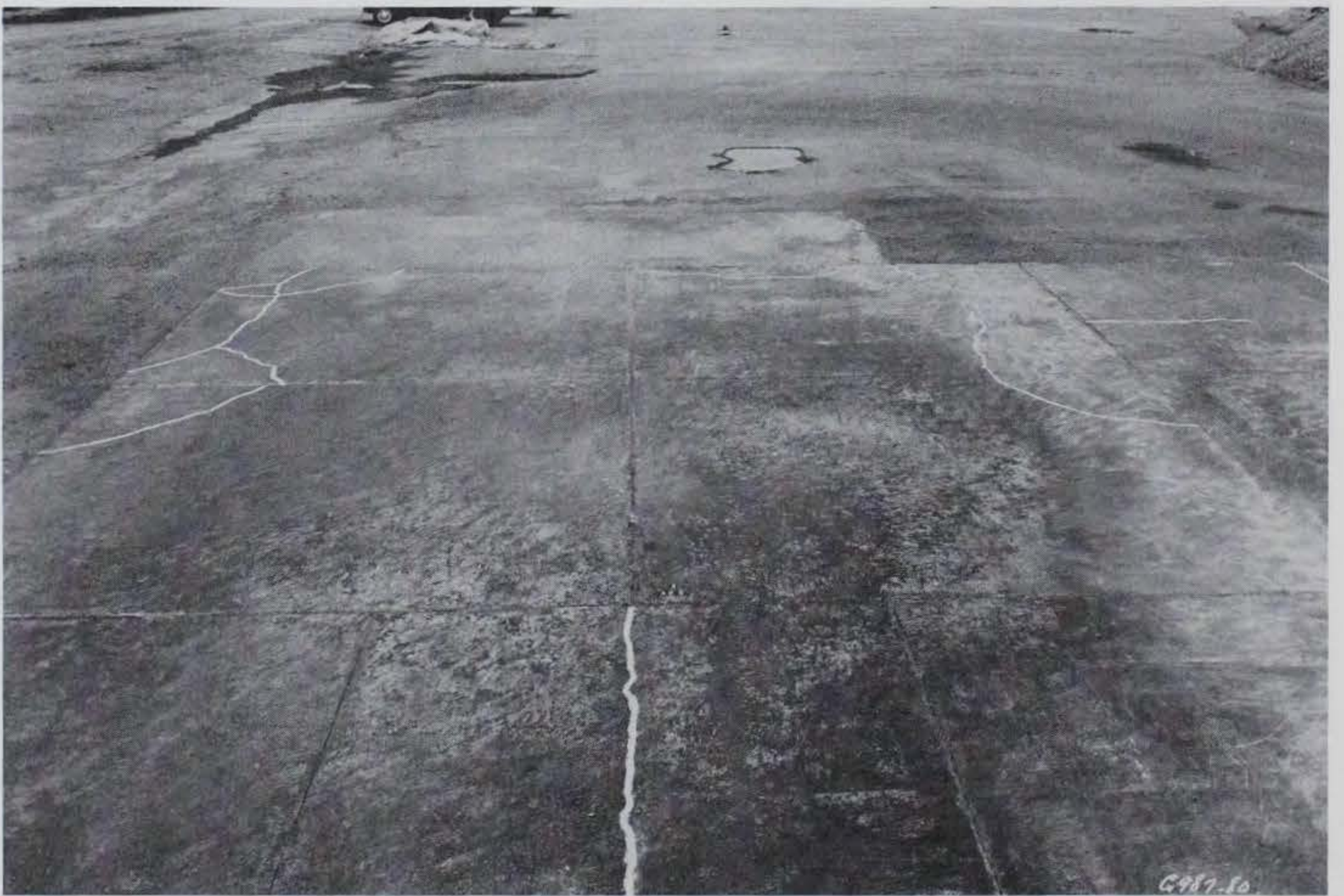
Photo 28. Item 5 after 2500 passes and 500 turning movements
