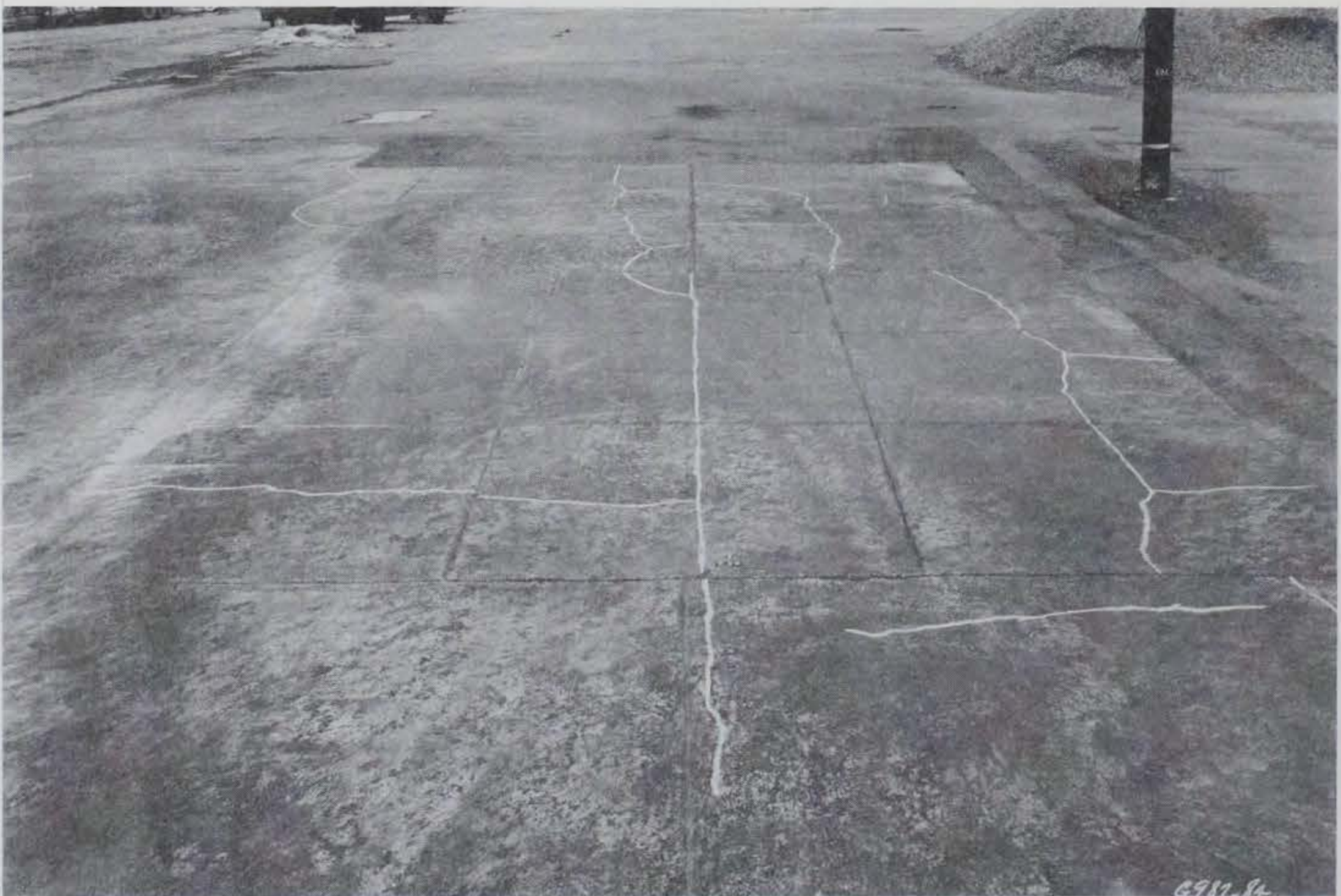
Photo 32. Item 9 after 2500 passes and 500 turning movements
