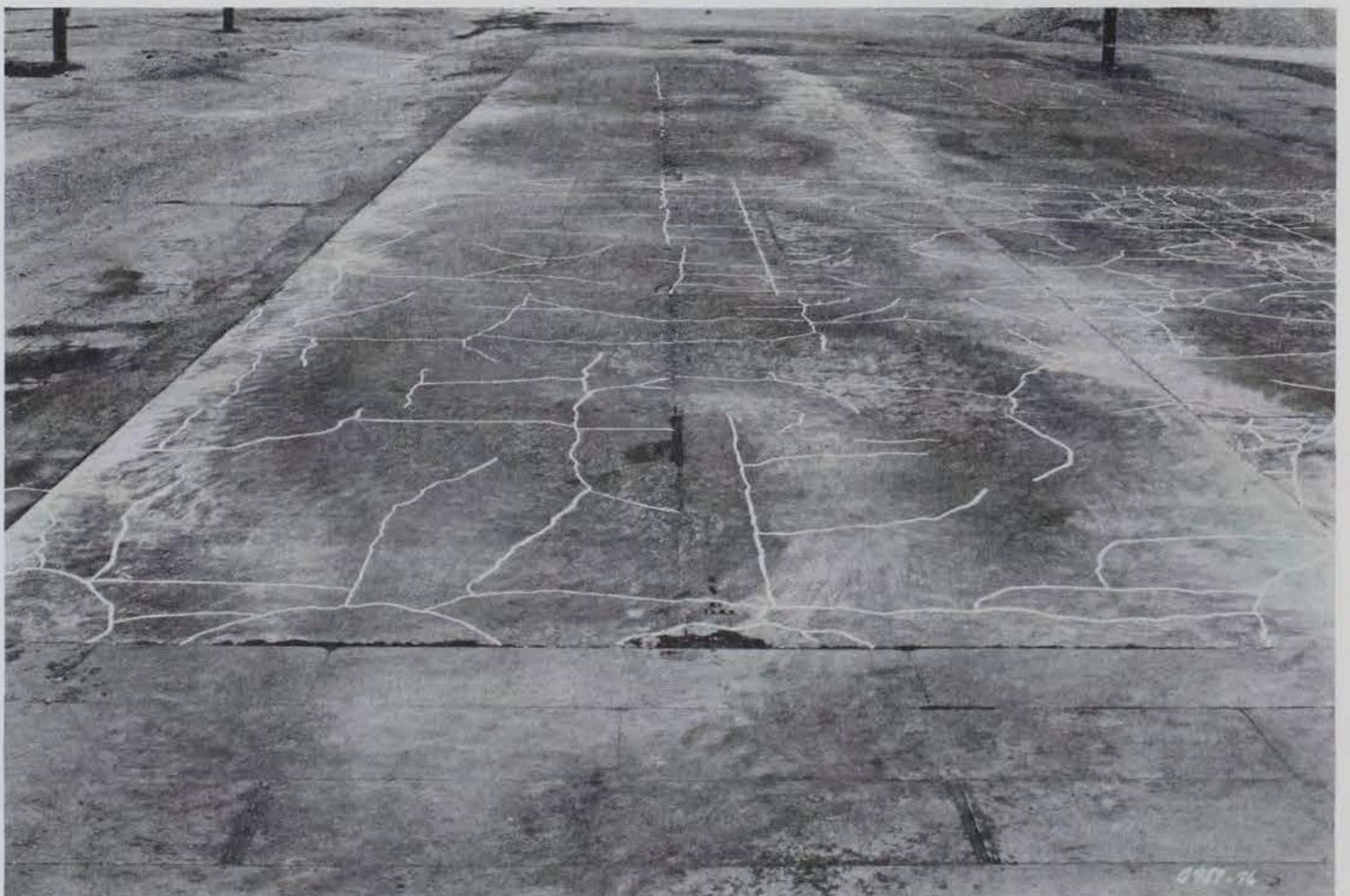
Photo 24. Item 1 after 2500 passes and 500 turning movements
