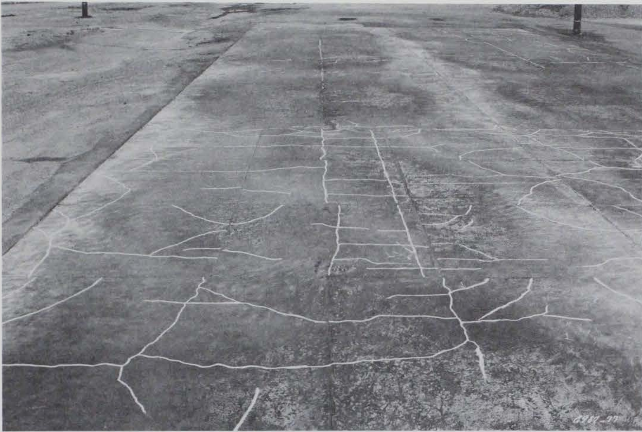
Photo 25. Item 2 after 2500 passes and 500 turning movements
