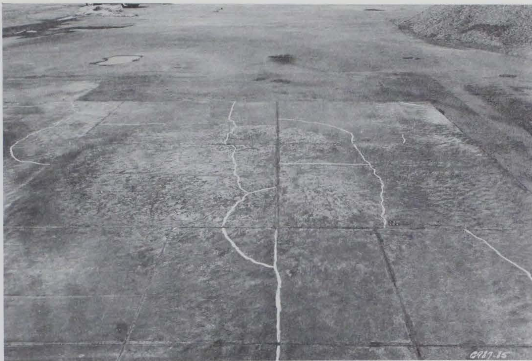
Photo 33. Item 10 after 2500 passes and 500 turning movements
