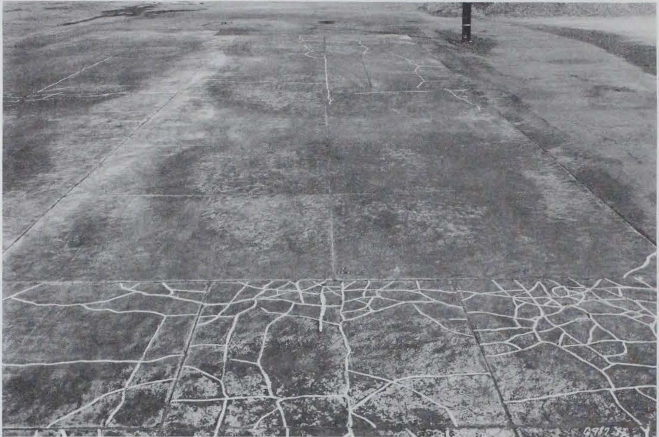
Photo 31. Item 8 after 2500 passes and 500 turning movements
