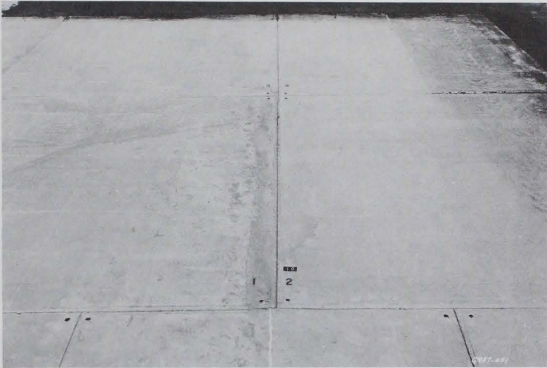
Photo 21. Item 10 before traffic
