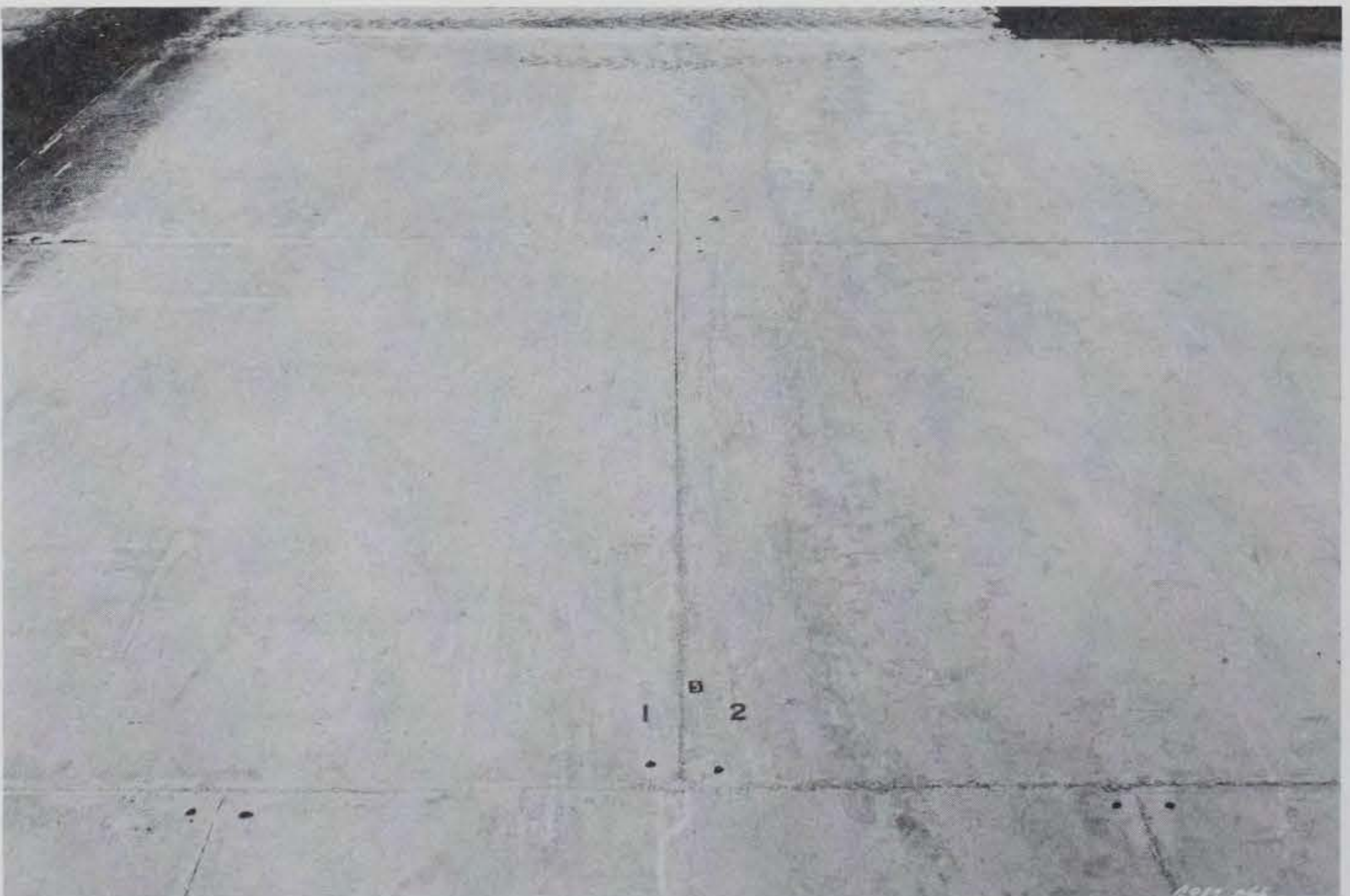
Photo 16. Item 5 before traffic
