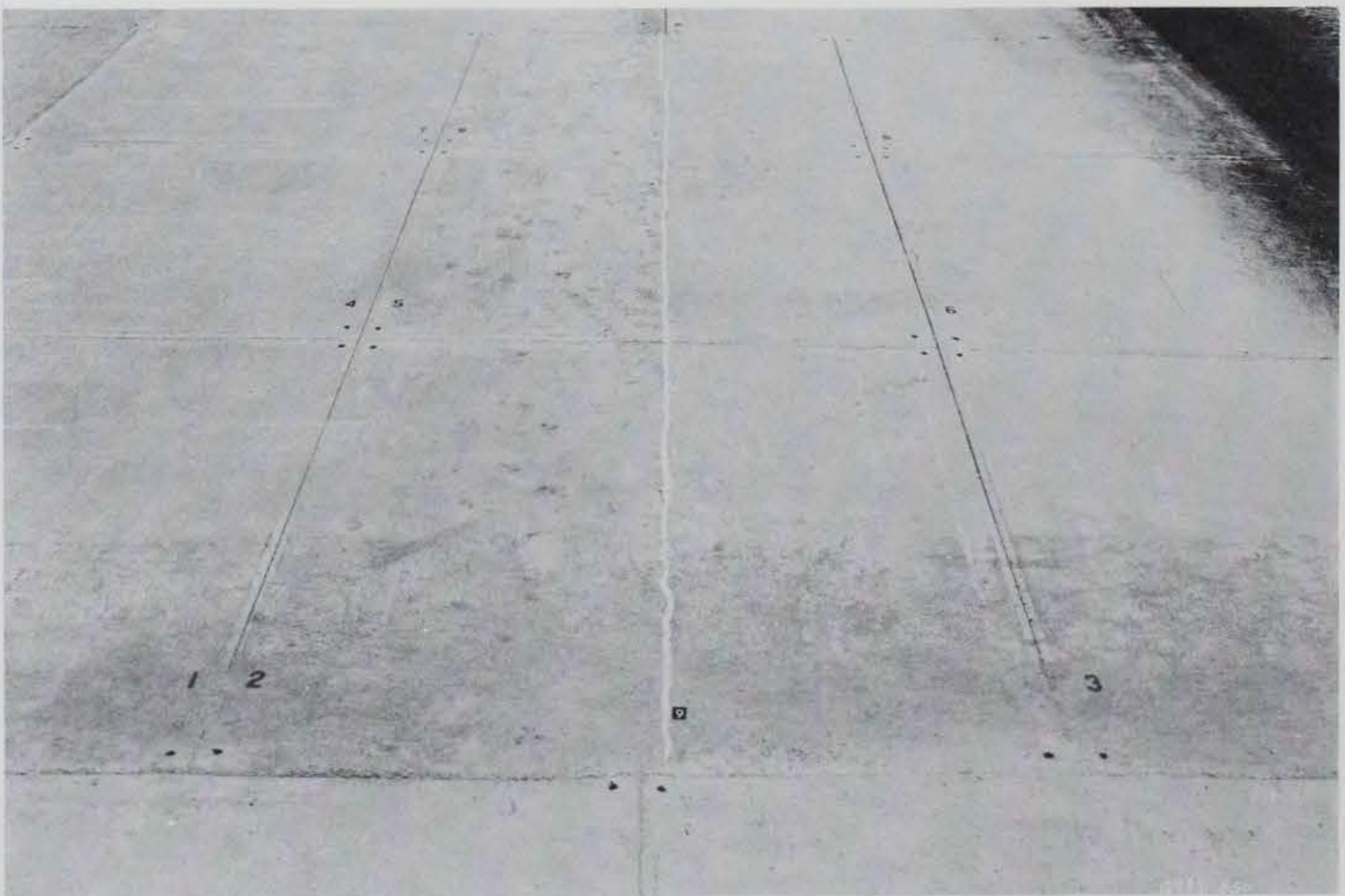
Photo 20. Item 9 showing a weakened plane progression crack from item 10
