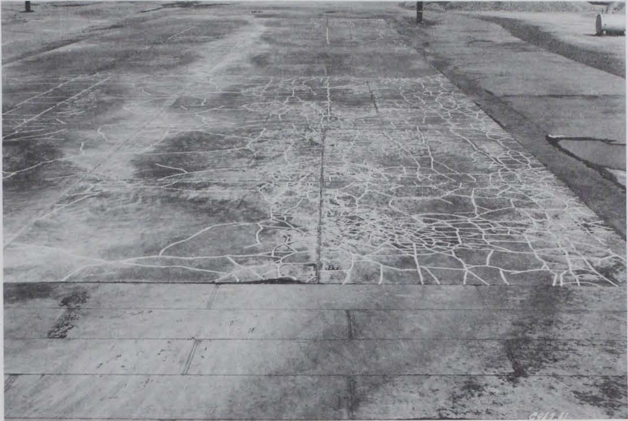
Photo 29. Item 6 after 2500 passes and 500 turning movements
