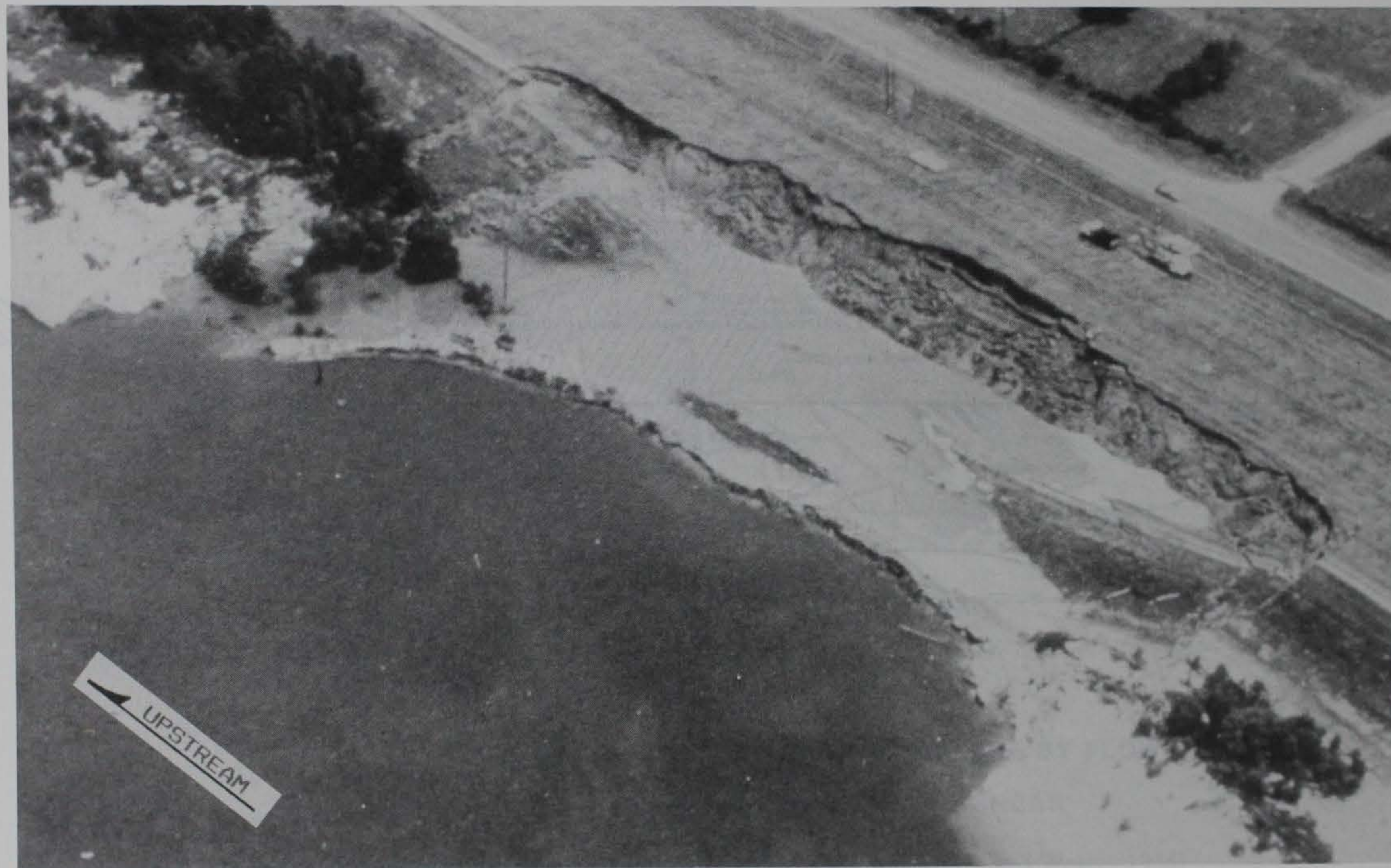
Figure 20. Aerial view looking upstream of the Marchand batture and levee failure
