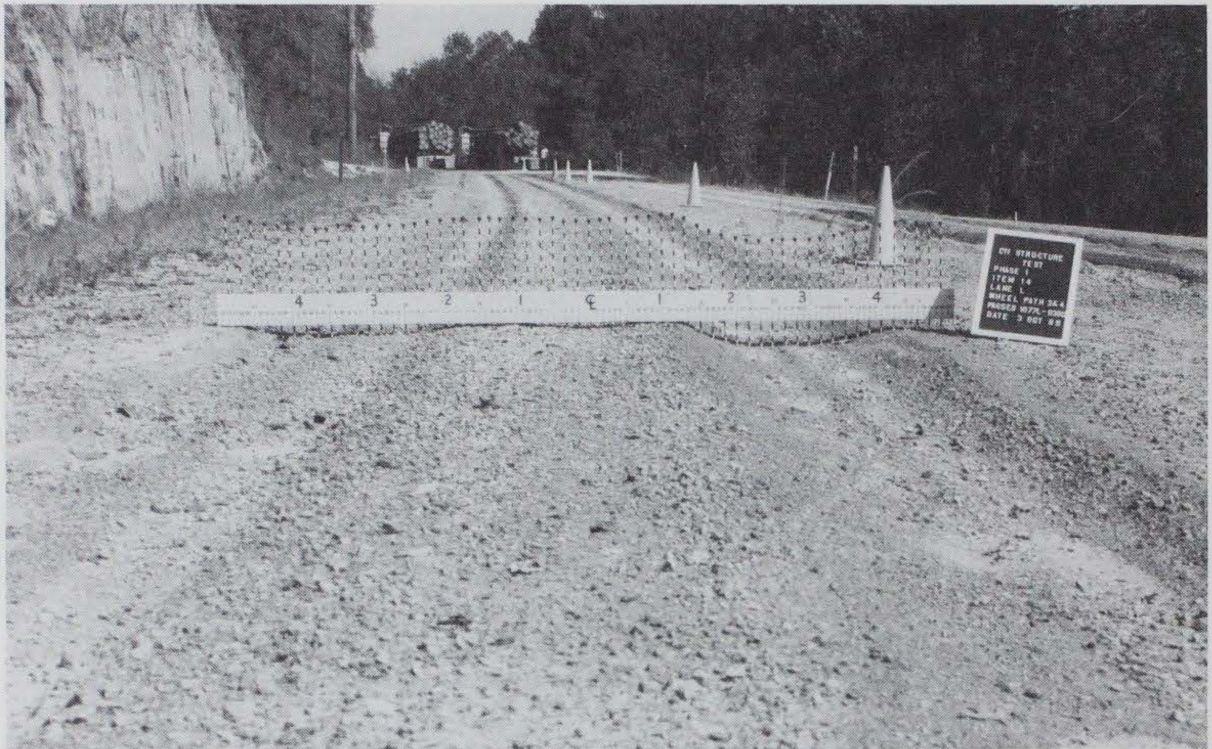
Figure 23. Low-tire-pressure lane, section 14, high-severity rutting after 90 passes in the rain
