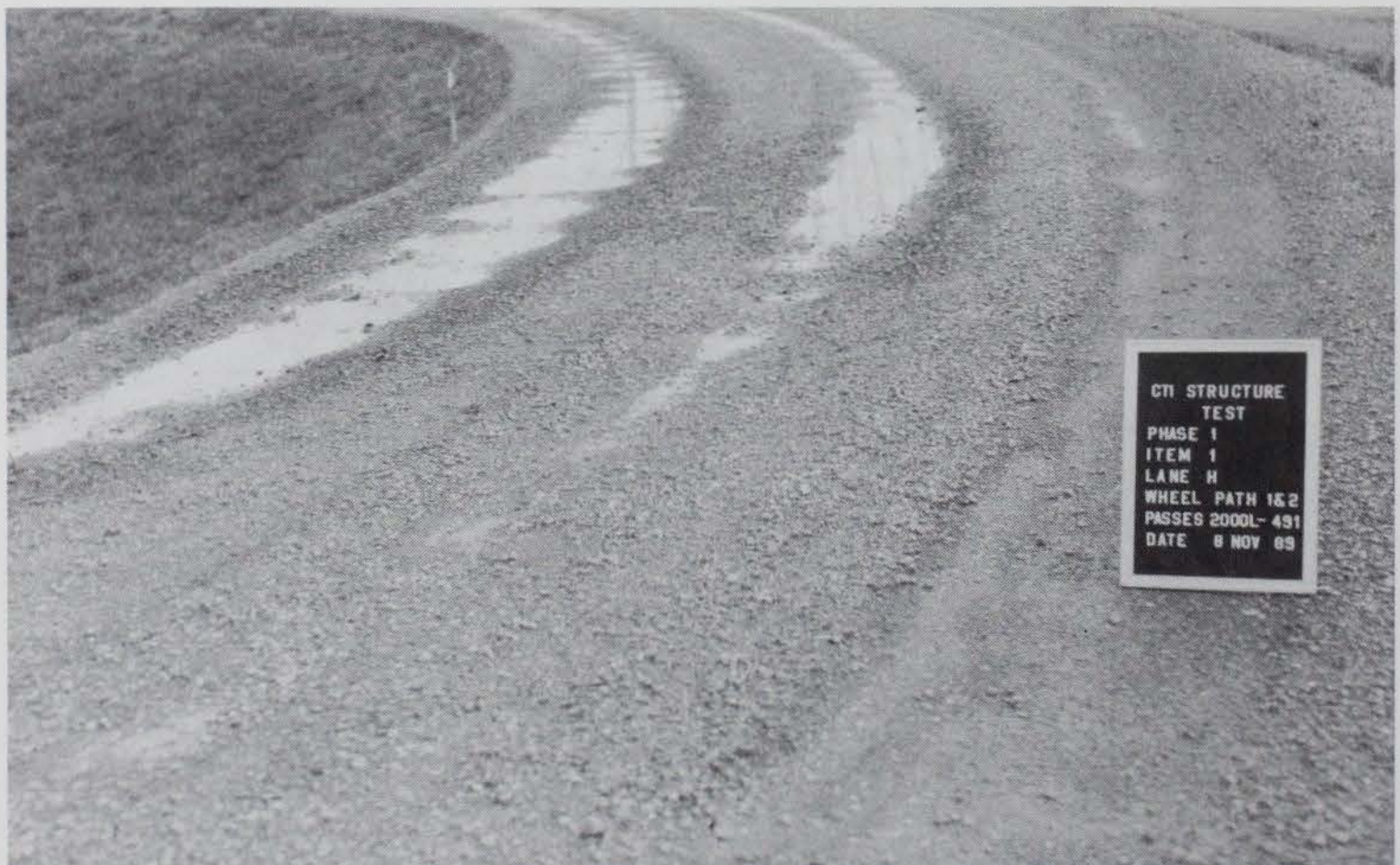
Figure 20. High-tire-pressure lane, section 2, low severity rutting and corrugation
