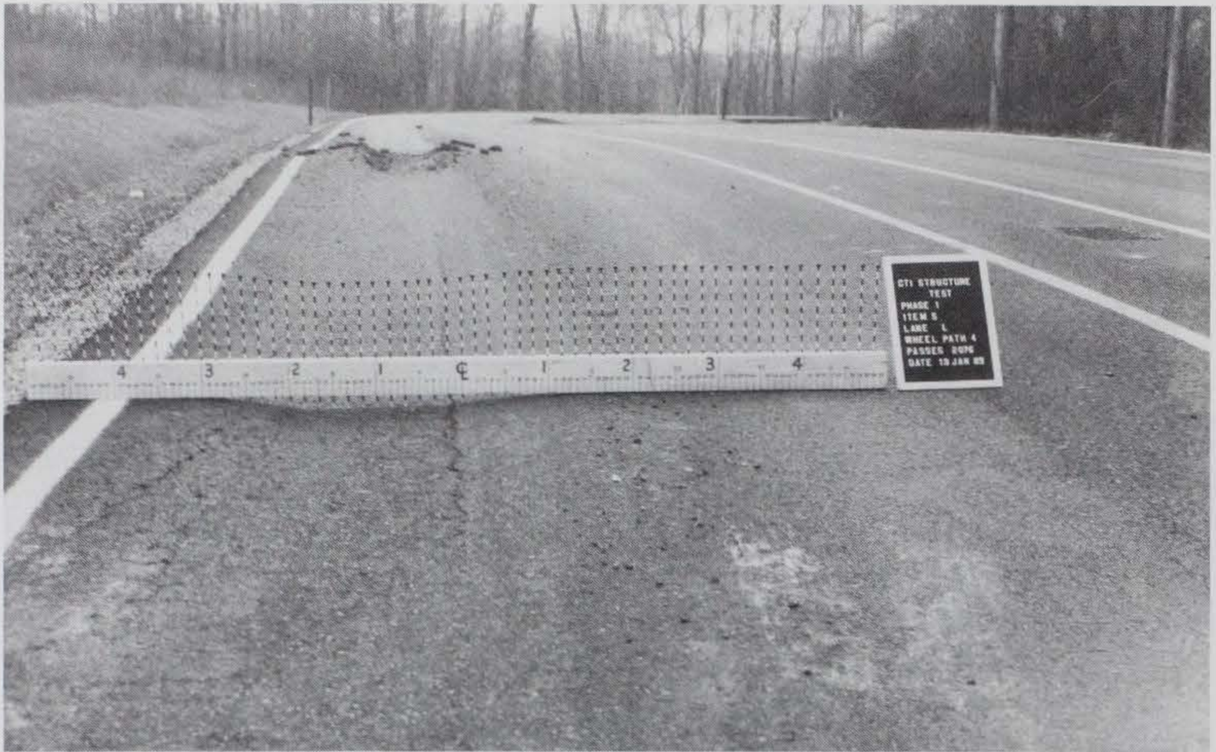
Figure 15. Low-tire-pressure lane, section 5, failure after 2,076 passes
