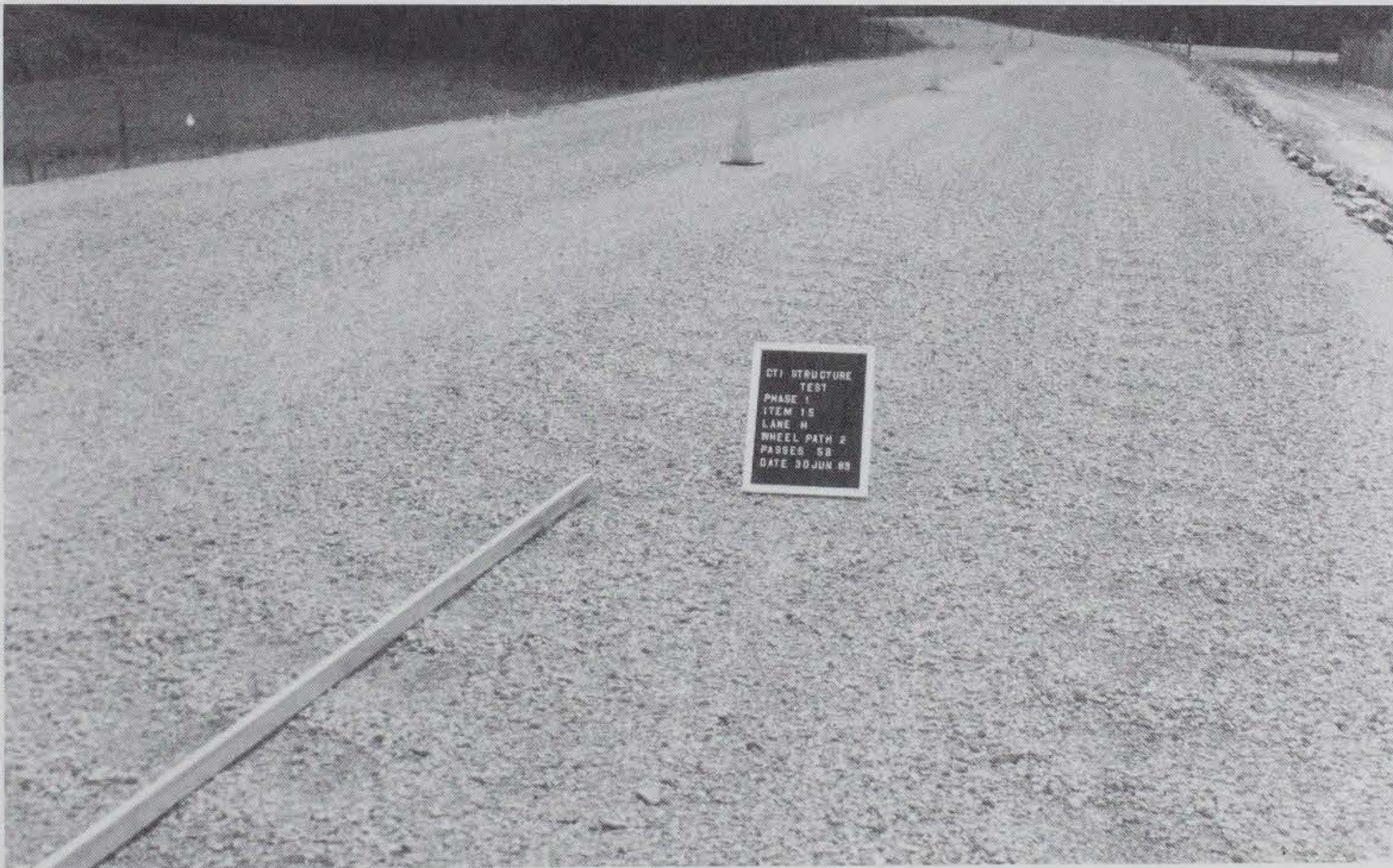
Figure 18. High-tire-pressure lane, section 15, low severity washboarding after 58 passes
