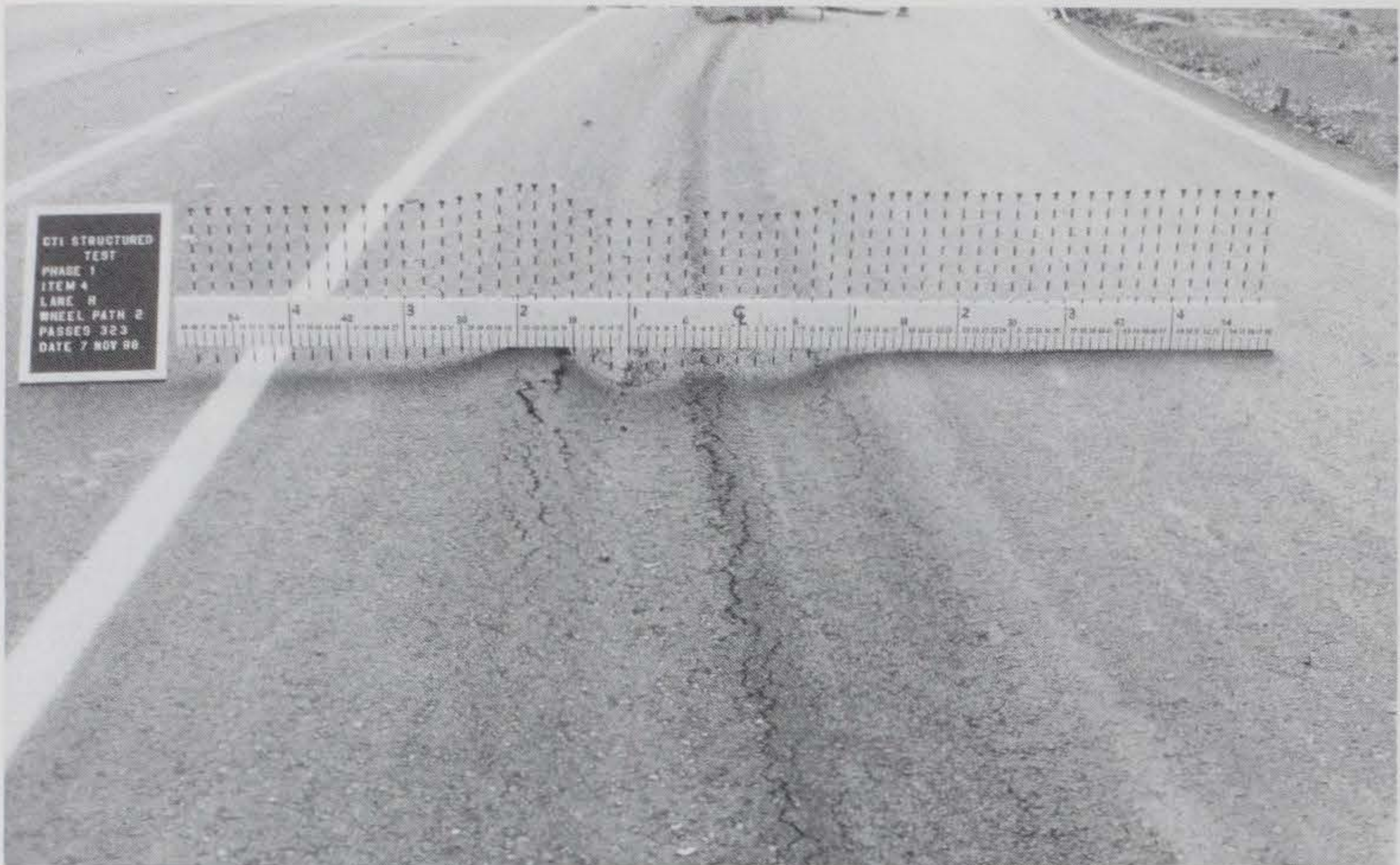
Figure 10. High-tire-pressure lane, section 4, second failure, 323 passes
